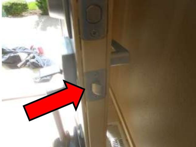
Door latch is not properly adjusted (sticks)
