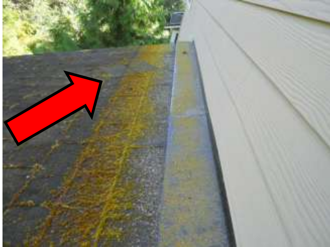
Moss build up on roof Shingles are lying on roof blown from other areas (see arrow)
