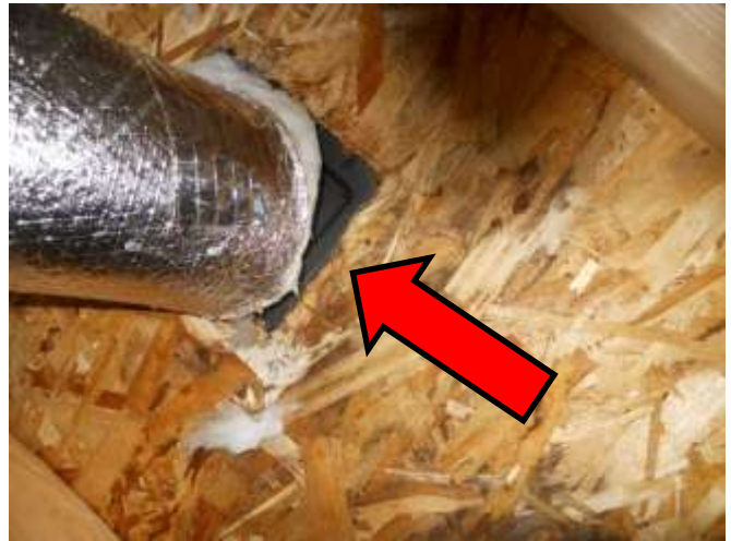
Dryer vent not properly secured
