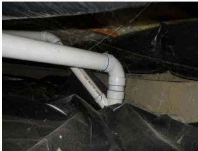
PVC Waste line in crawlspace
