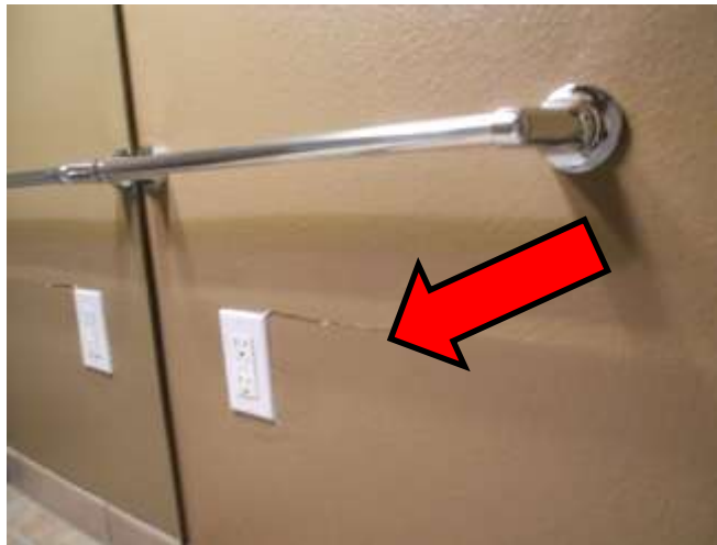
Minor drywall and backsplash damage from apparent moisture intrusion from attic. See Building Exterior section
