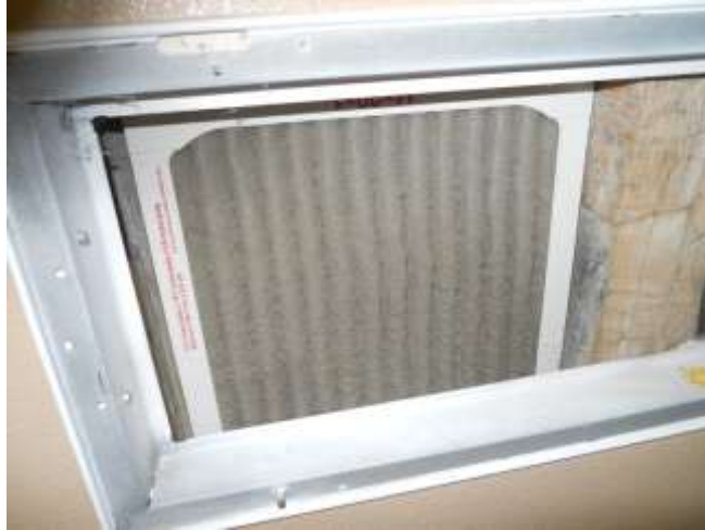
Furnace filter is very dirty
