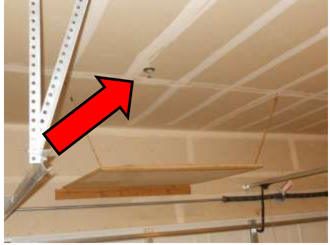
Storage above garage door near fire control head
