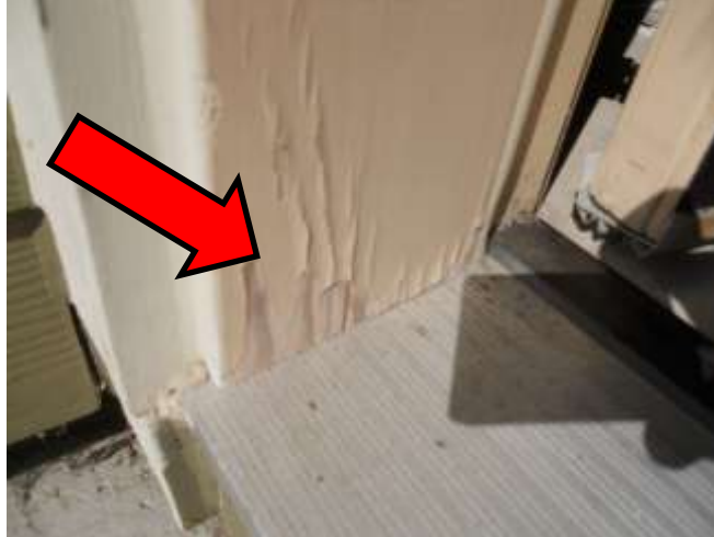
Exterior door jambs should be maintained as they are the most susceptible to wood rot
