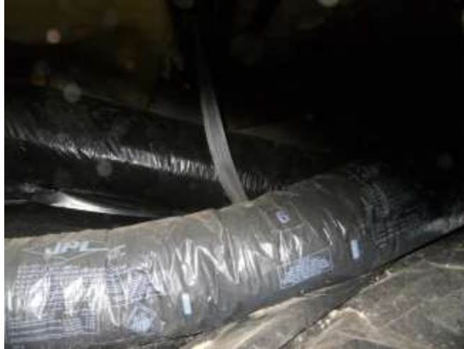
Heat ducts lying on ground
