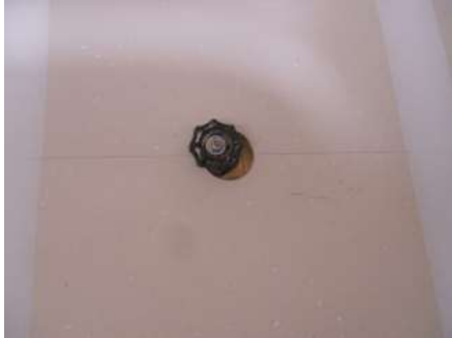
Winter shut off for front hose bib located in garage
