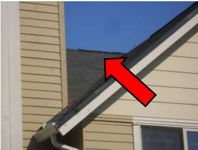
Ridge shingles missing
