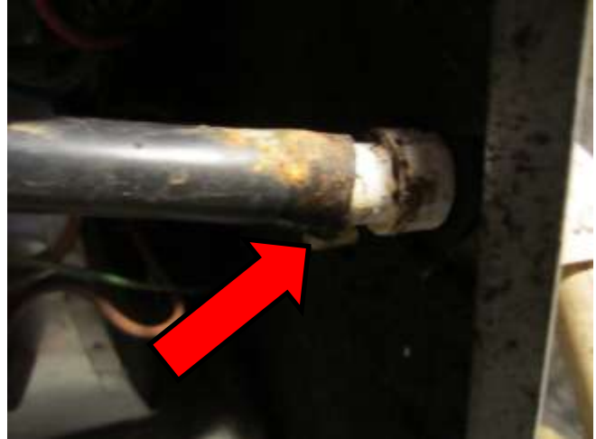
Leak at condensation line
