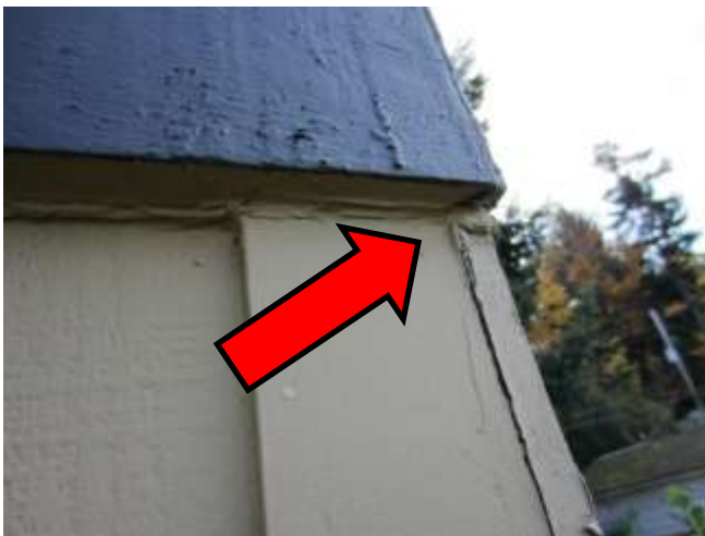
Impropr flashing at S.W coner of Master bedroom
