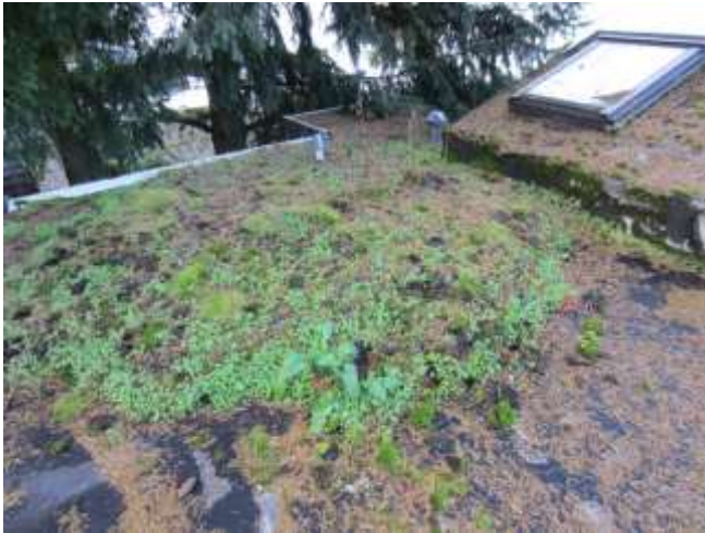
8" + of debris on roof
