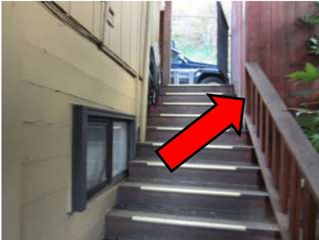
Graspable handrail not installed
