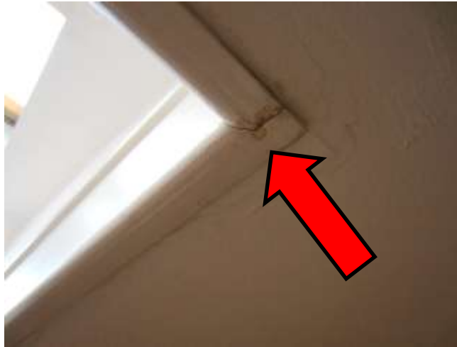
Moisture stains at skylight well trim
