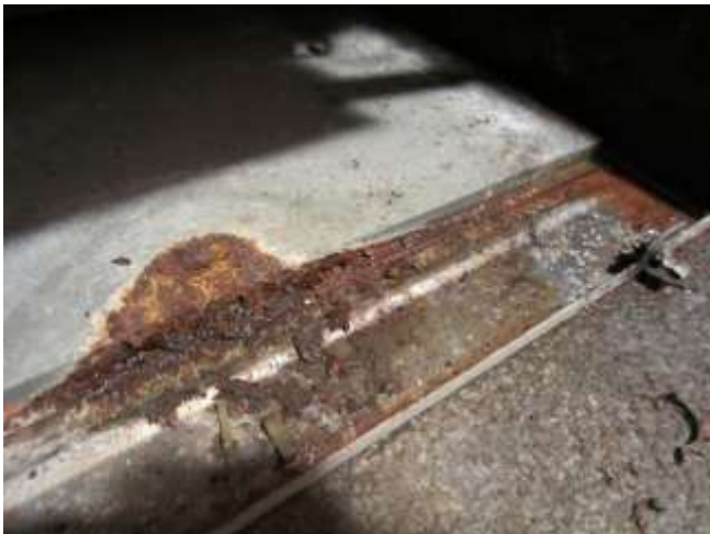
Rust at base of furnace
