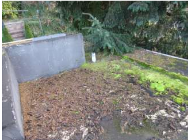
Debris on roof
