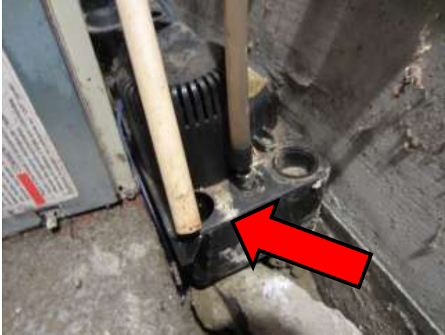
Condensation line not connected to pump
