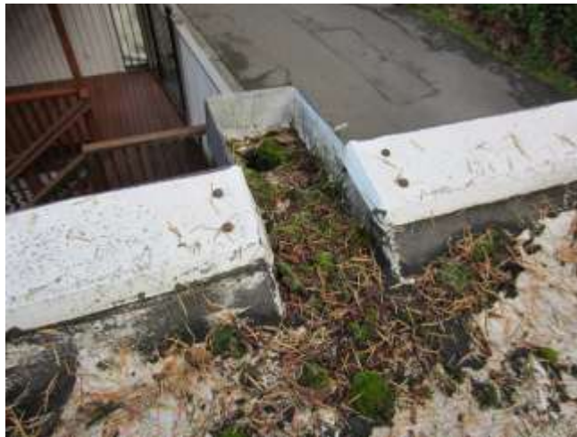
Debris in scuppers
