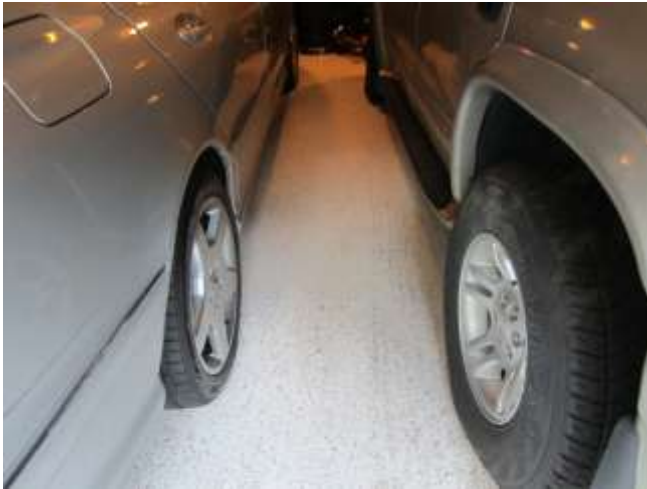
Garage slab appears to slope towards the house
