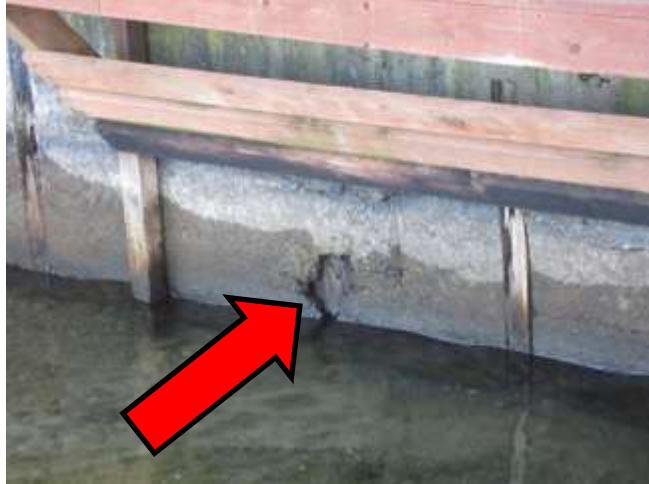
Deterioration at bulkhead
