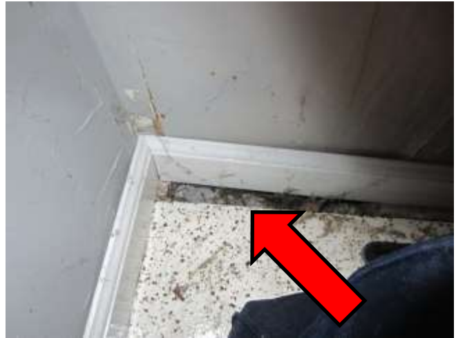
Gap at garage slab adjacent to house
