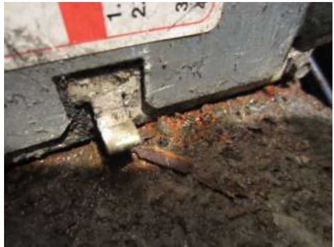
Moisture from base of furnace
