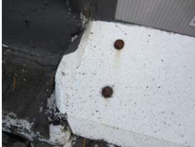
Rusting flashing nails These nails should be coated to prevent moisture intrusion
