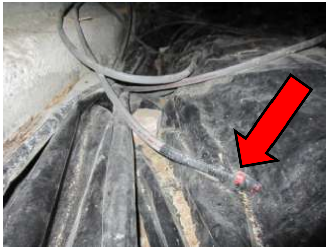
Loose wire in crawlspace
