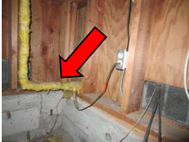
Pipe heating tape at S.W. area of crawlspace
