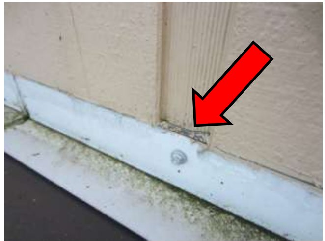
Caulking at vertical grooves must be maintained
