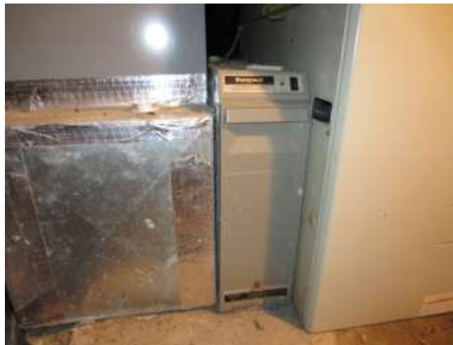
Furnace filter location
