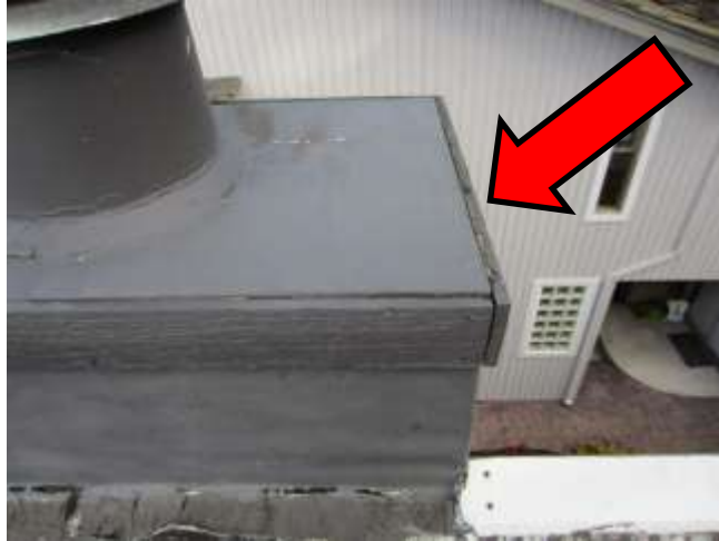
Flashing not installed at chimney cap trim
