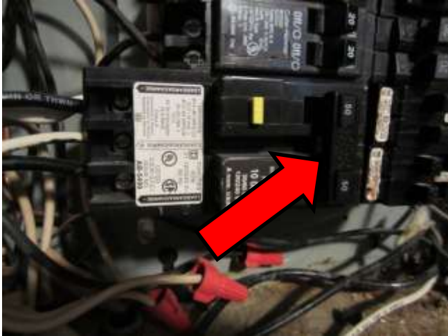
Dock GFCI will not reset Test GFCI once operational
