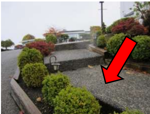
Walkway leans towards driveway
