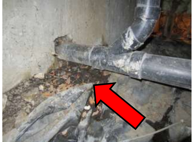
Moisture intrusion at sewer discharge pipe
