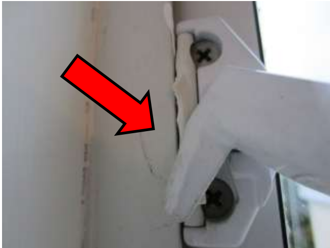
Deteriorated window hardware
