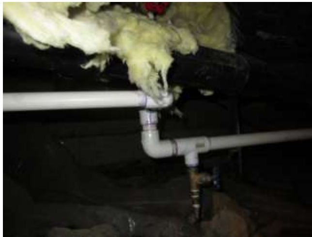
Pipes and valves near the crawlspace access
