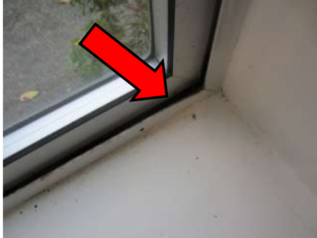
Large gaps at base of casement windows
