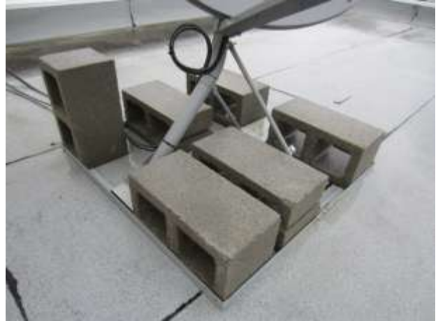
Concrete block to secure dish antenna
