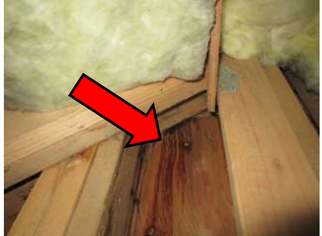
Moisture (wet) below stairs to game room
