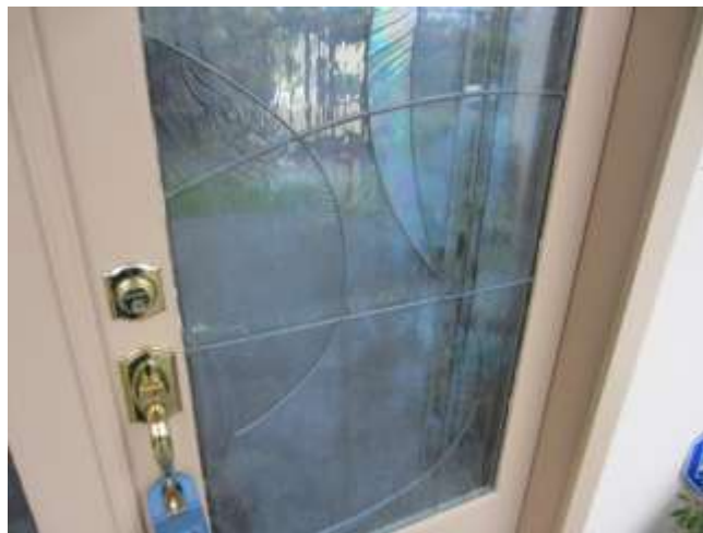
Failed from door glazing (fogging)
