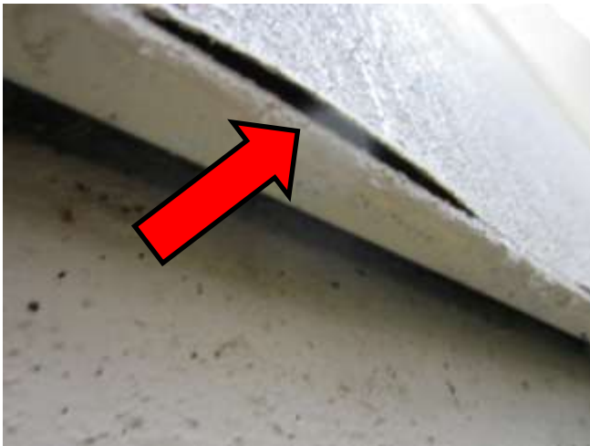
Separation of stucco finish
