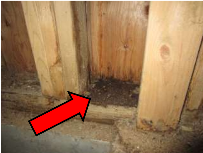
Moisture (wet) below stairs to game room
