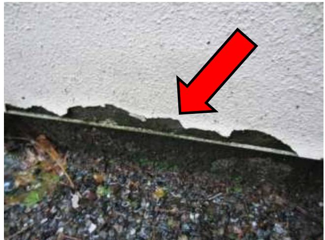
Deterioration of stucco at base
