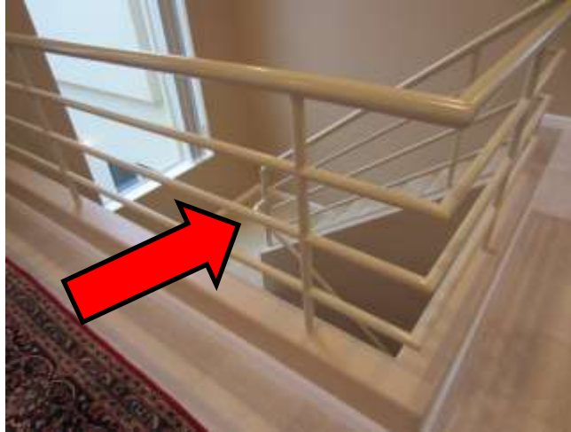
Horizontal balusters create a ladder and subsequent fall hazard for children
