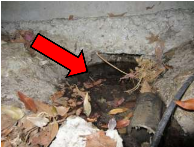
Moisture intrusion (flowing water) from behind the garage. Water flows to a sump pump
