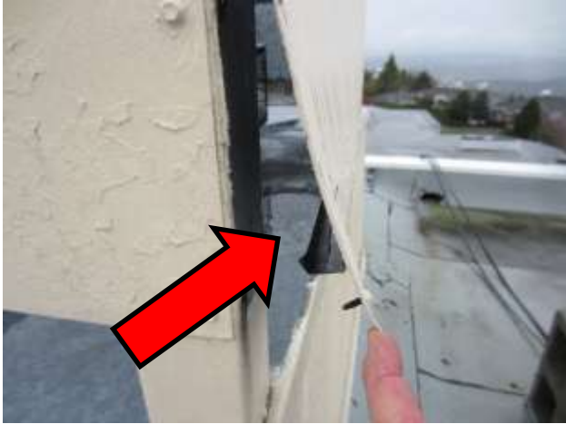
Separation at fireplace shroud
