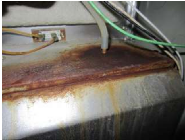
Rust on top of combustion compartment
