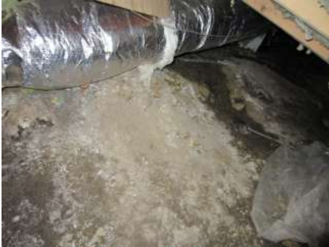
Exposed ground (no vapor barrier)
