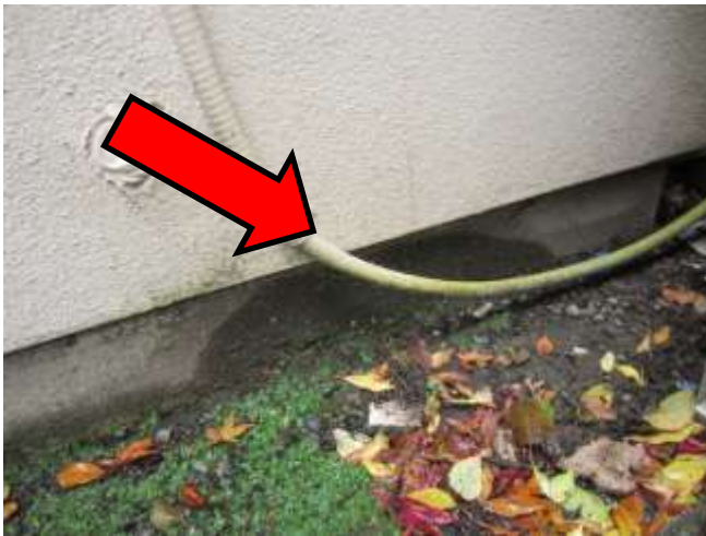
Moisture stain at foundation wall Stain is located beneath rear stair stringer This moisture may be ground “splash-back” related as the top of the stain is arced (not vertical)
