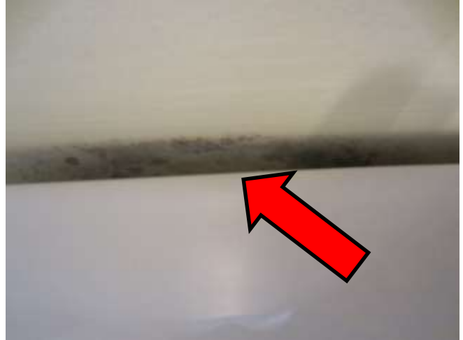
Evidence of microbial growth behind toilet lid
