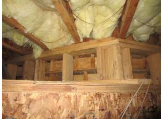
No insulation at rim joist
