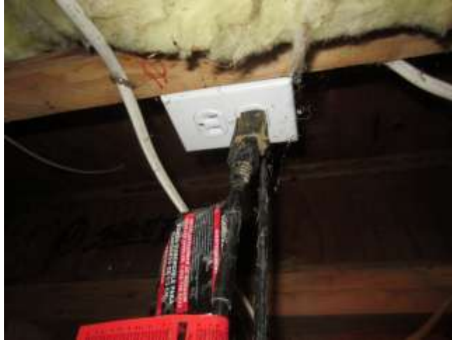
Sump pump should be GFCI protected
