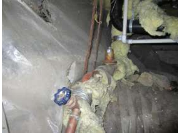
Domestic Water Shut off
