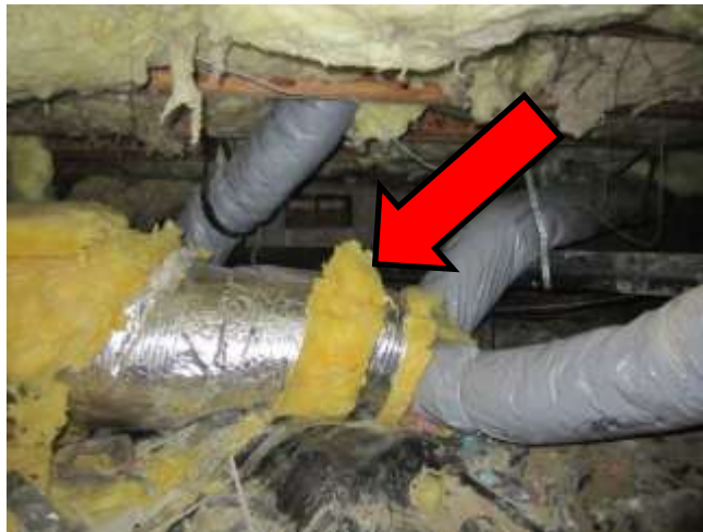
Heat ducts are not secured to floor joists above
