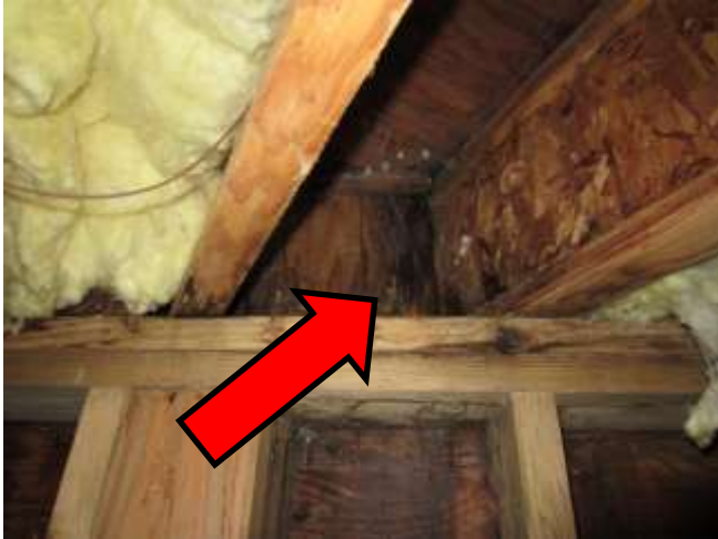
Moisture stains and (wet) wood rot below the rear deck
