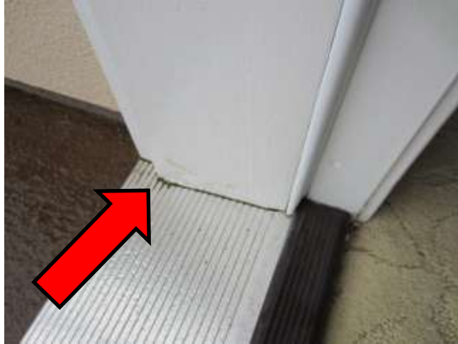
Minor wood rot at door jamb
