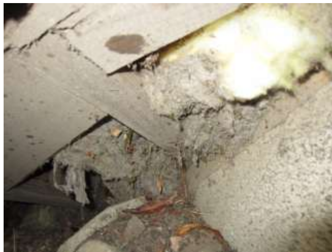
Exposed insulation below Living Room cantilever
