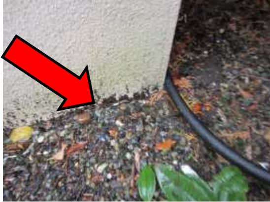
Siding in contact with ground
