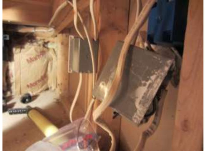
Unsecured wires and boxes at spa access
