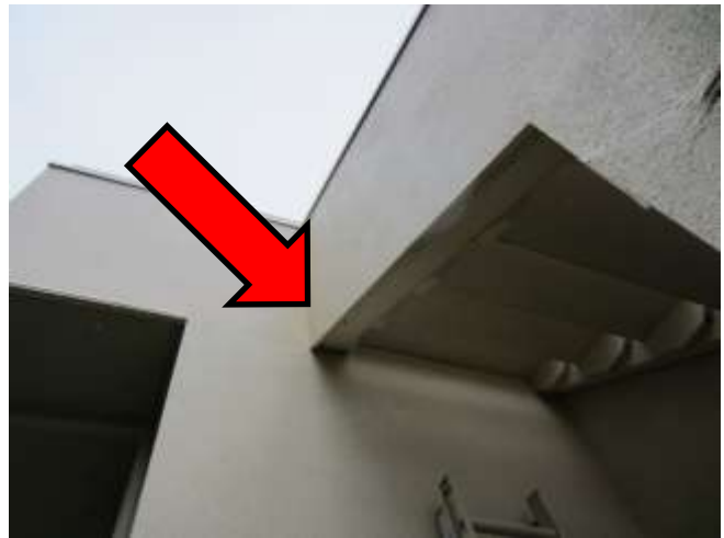
See image to left Stain is located beneath this area
