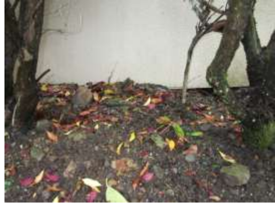
Dirt piled up in contact with living room cantilever
