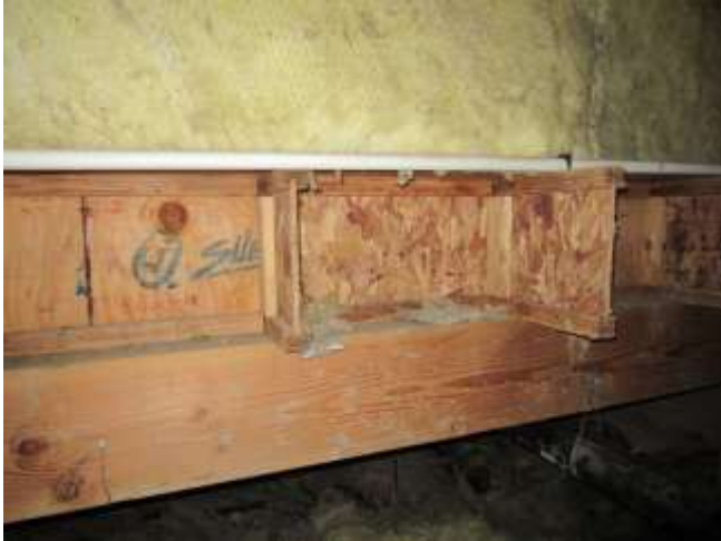
No insulation at rim joist
