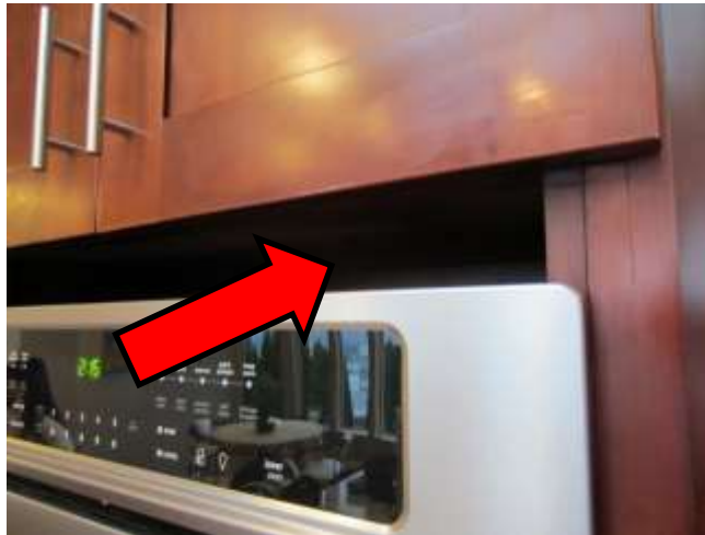
Large gap above oven
