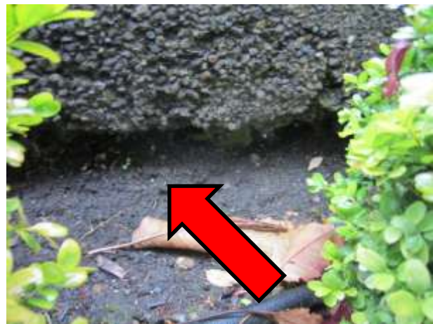
Walkway is not supported in certain areas
