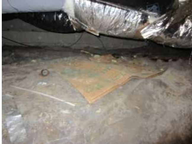
Cardboard debris in crawlspace
