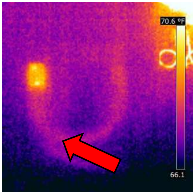
Electrical wires to thermostat
