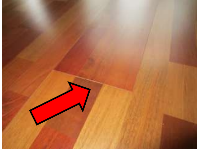
Edges of laminate hardwood are not flush
