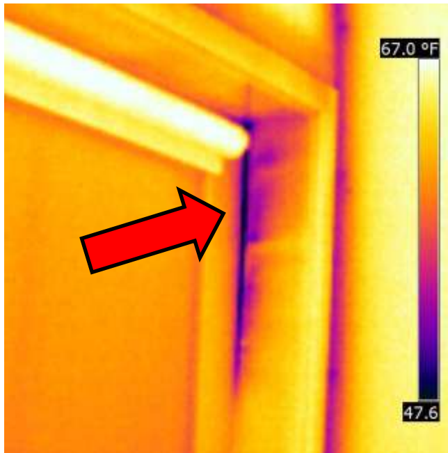
Air leakage at the door to the deck
