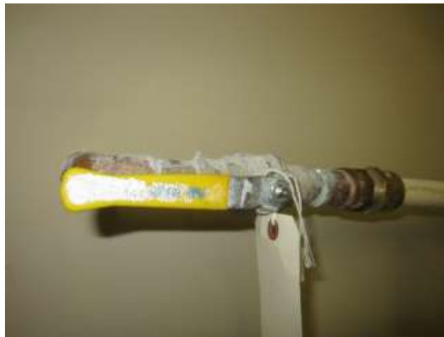
Domestic water shut off
