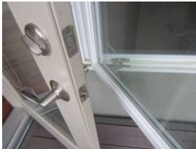
Window conflicts with deck door
