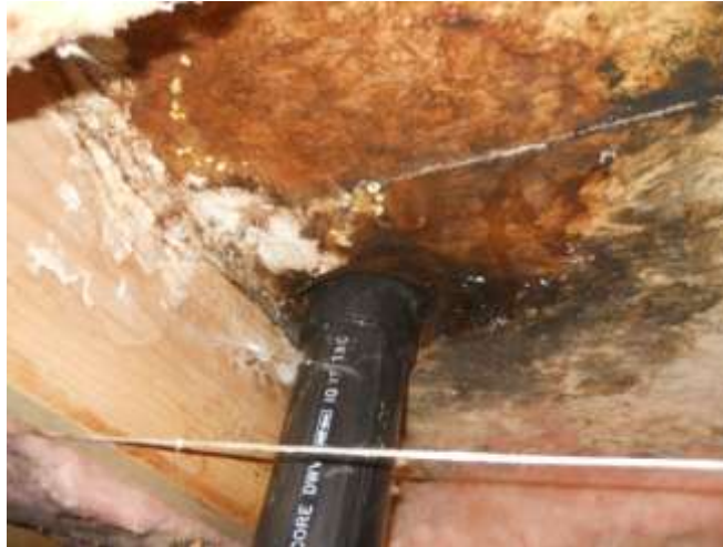
Moisture damage below Master bathroom
