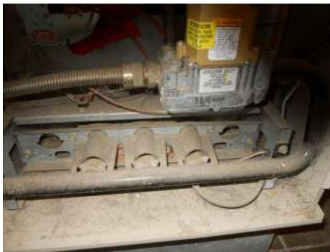
Dust and lint in burner area
