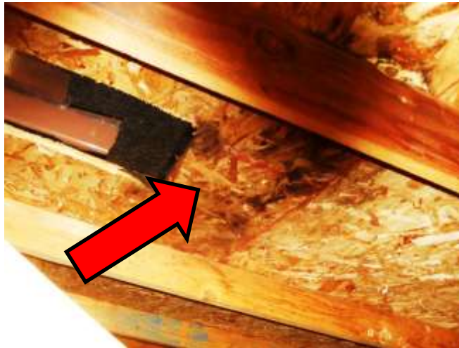
Wood rot at sheathing below roof jack
