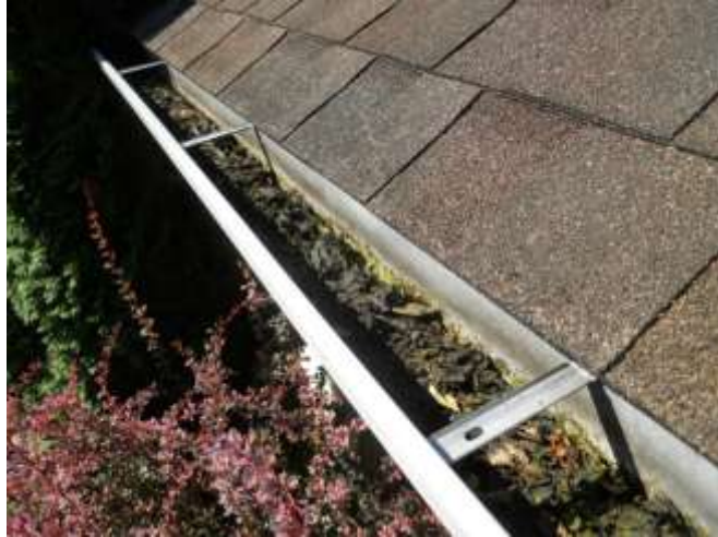
Debris in gutters (typical)
