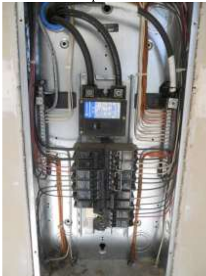
Service panel: garage
