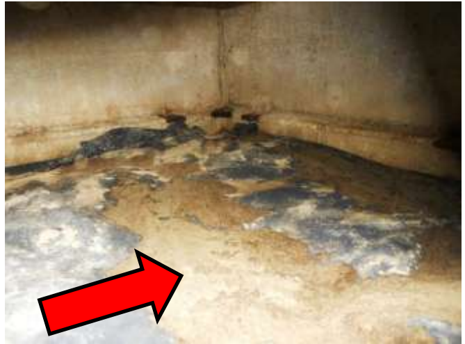
Mud trail beneath corner of addition by deck
