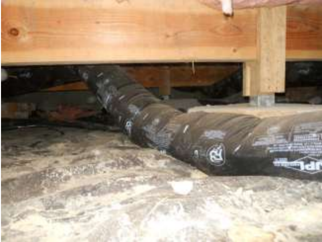
Heating duct lying on ground
