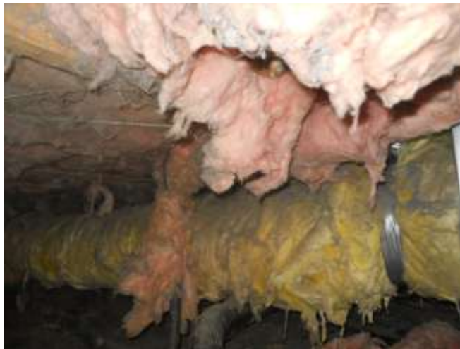
Substantial lint in crawlspace near dryer vent
