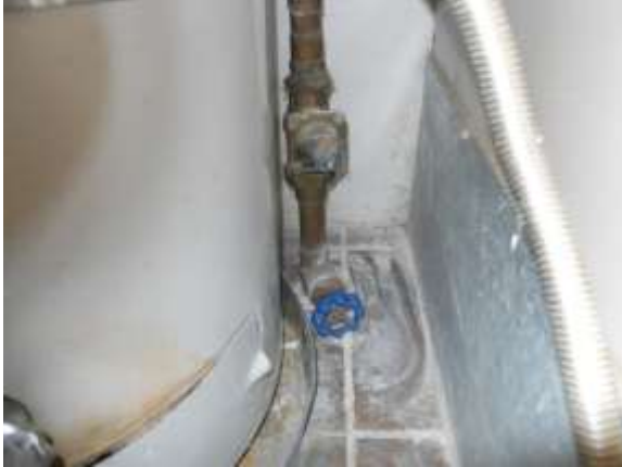
Domestic Water Shut off at house
