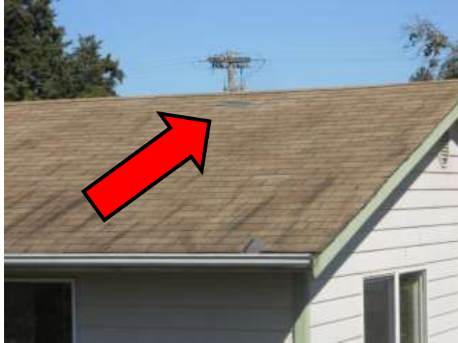
Shingles missing at roof
