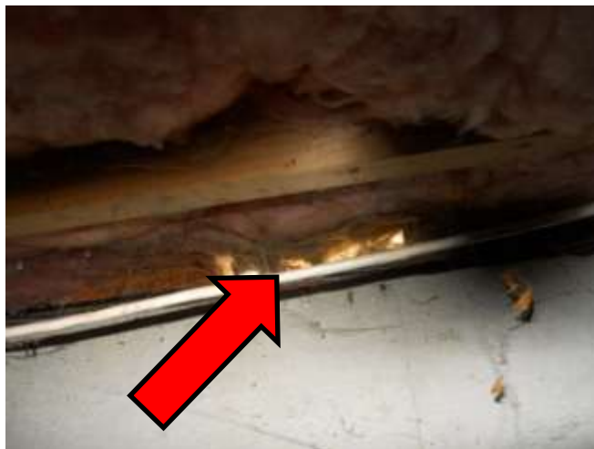
Partially obstructed foundation vent at original house
