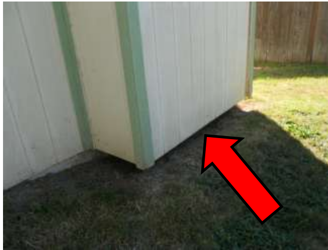
Insulation and soffit not installed
