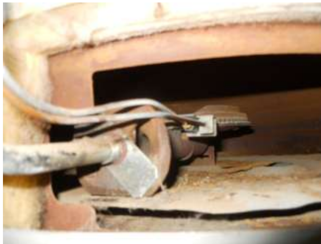
Rust in burner compartment
