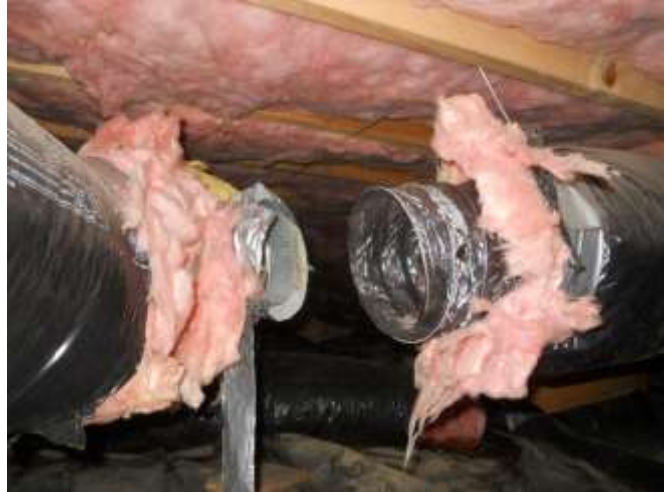
Heat duct disconnected from trunk line
