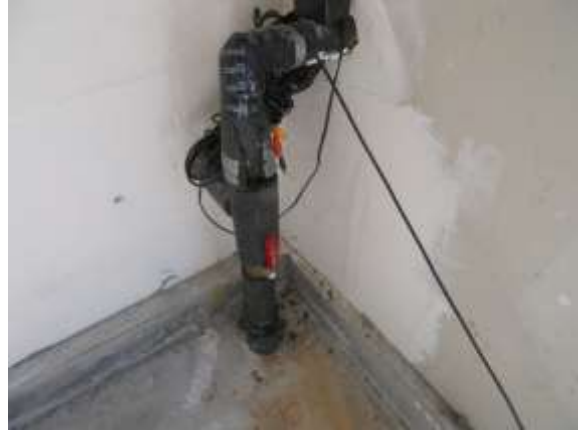
Domestic Water Shut off at garage
