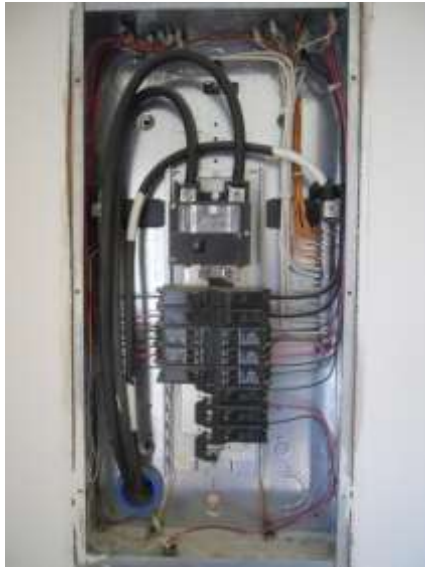
Service panel: House
