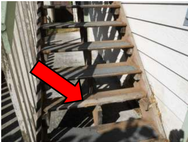
Broken stair tread (typical)
