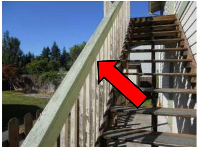
No graspable handrail
