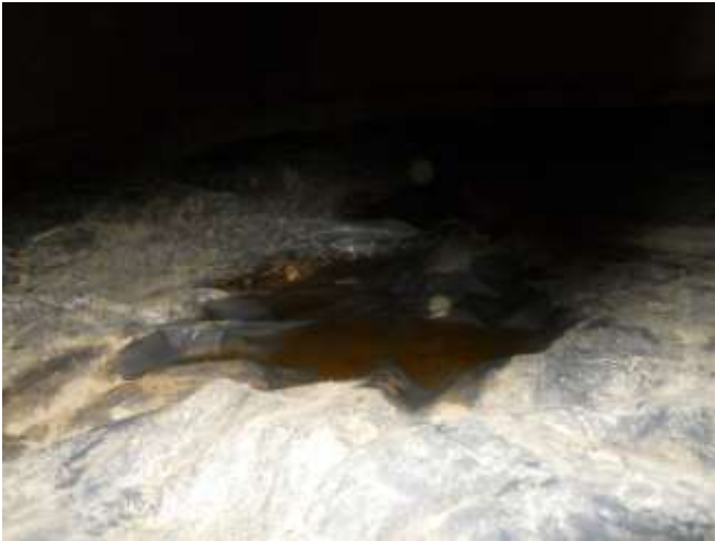
Standing water in addition area
