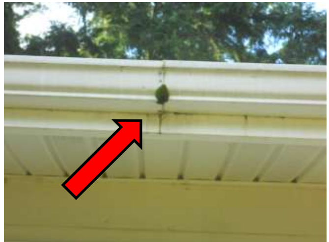
Evidence of gutter leak
