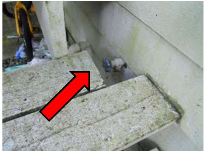
Trip hazard at hose bib
