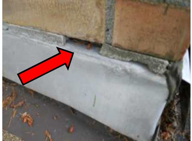
Missing mortar at chimney
