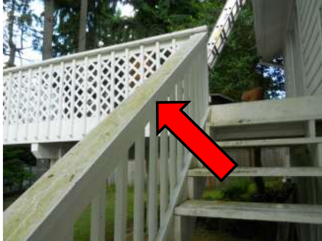
Graspable handrail not installed
