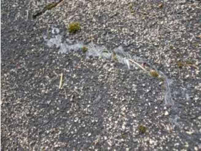
Worn shingle (typical)
