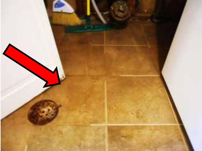
Waste water flowing out of floor drain
