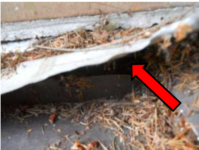
Gap at chimney flashing
