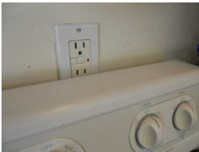
Electrical outlet above range is a safety hazard
