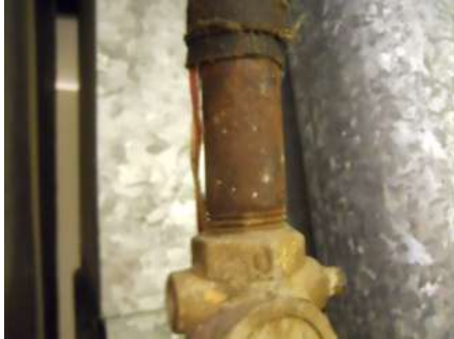
Extensive rust at gas pipes
