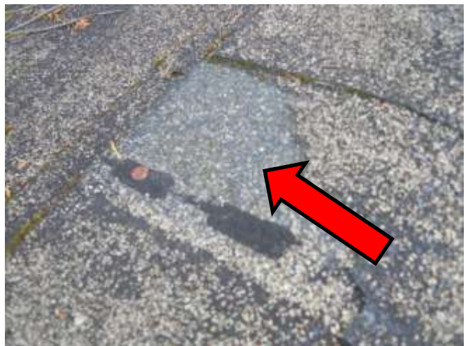
Missing shingle (typical)
