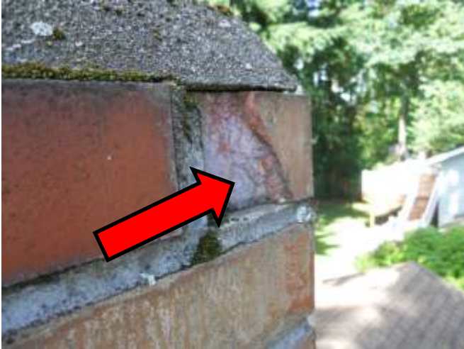
Cracked chimney brick
