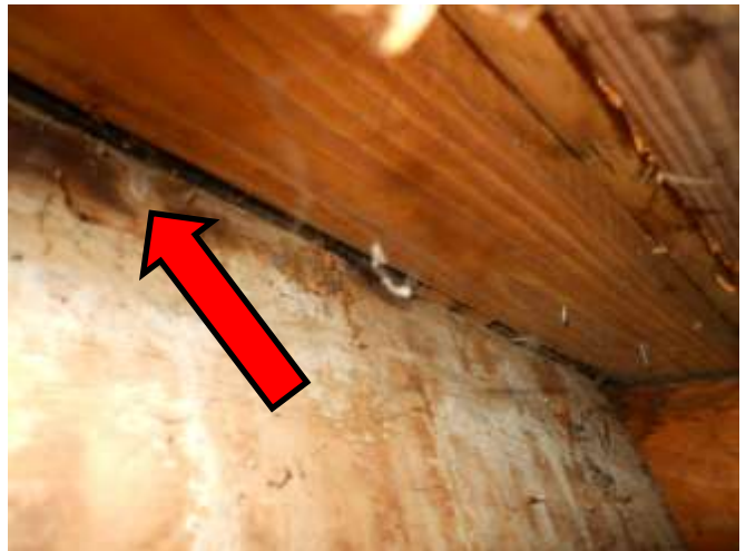
Moisture at attic ridge beam
