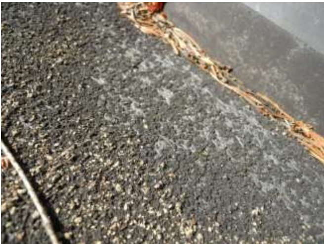
Worn shingle (typical)
