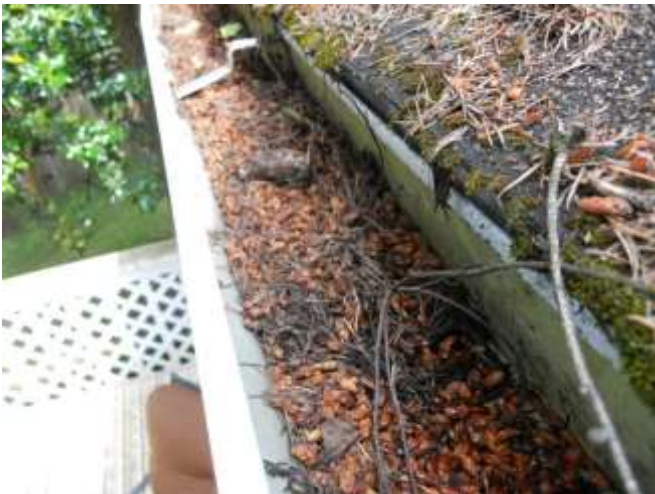
Debris in gutter
