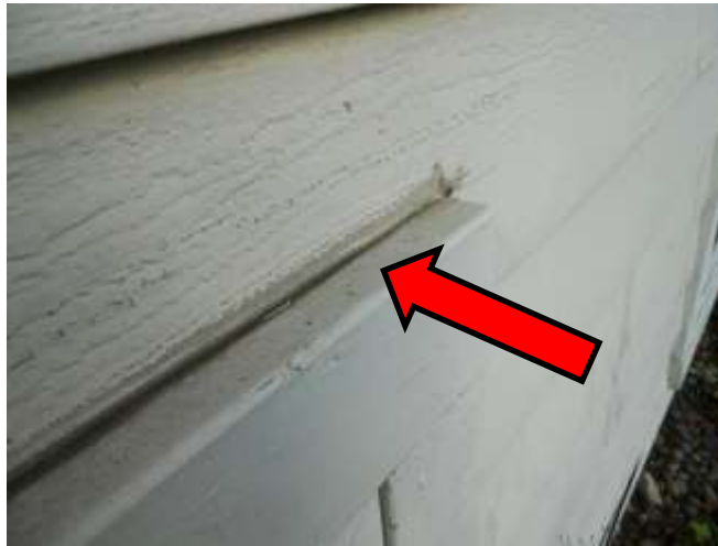
Flashing not installed at window trim
