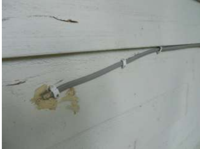
Power supply to garage should be in conduit
