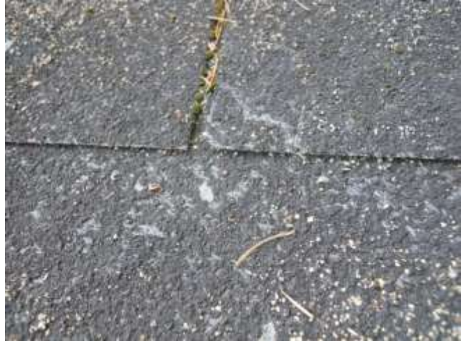
Worn shingle (typical)
