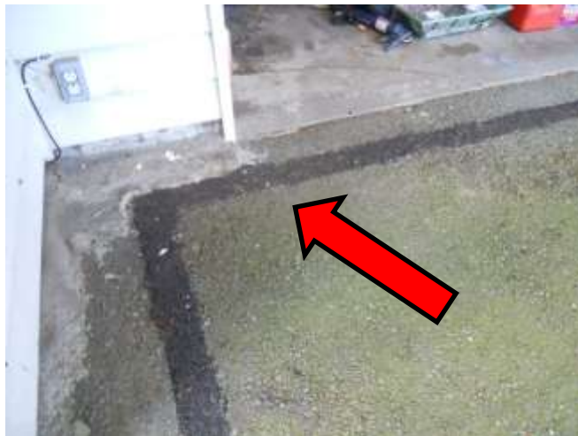
Unknown purpose of repair to driveway near garage
