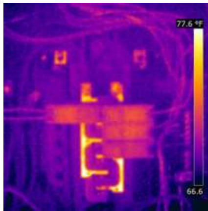
No evidence of overheating
