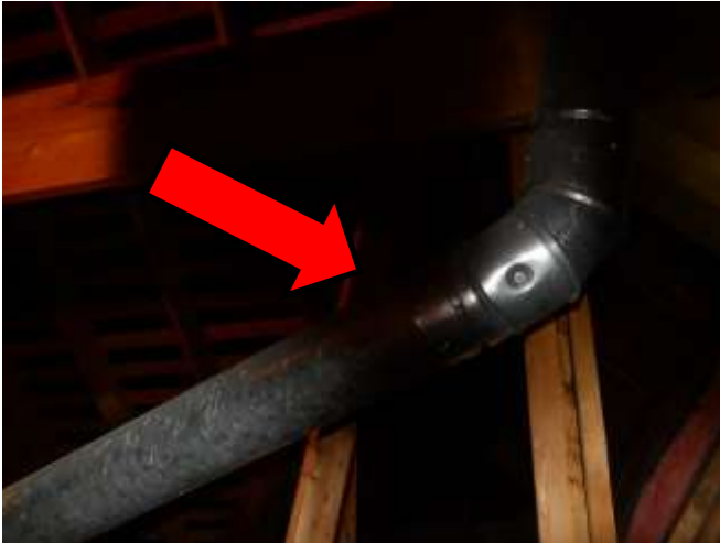
Un-supported furnace flue
