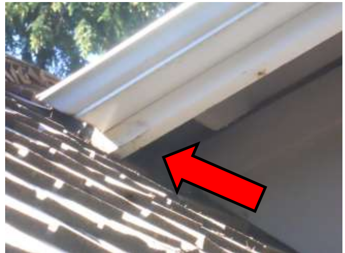
Blocking may be missing at game room (leads to bird nesting)
