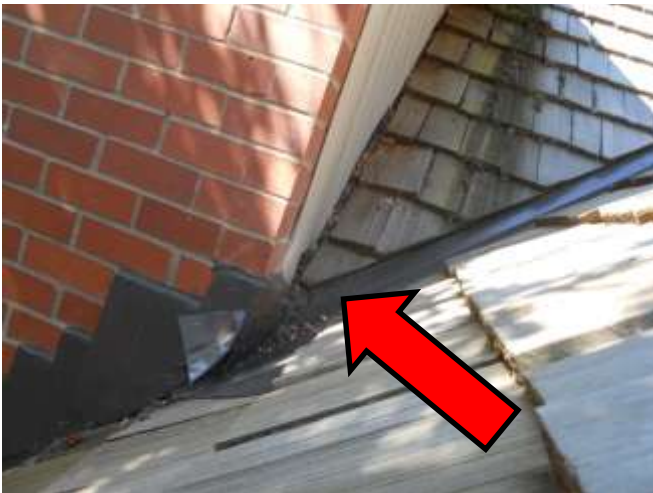
Valley at left side of entryway must be kept clear of debris
