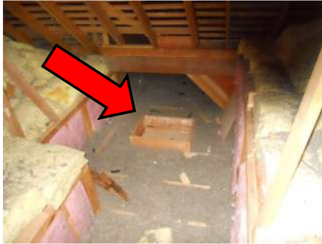
Lower attic access at Master Bedroom is not insulated
