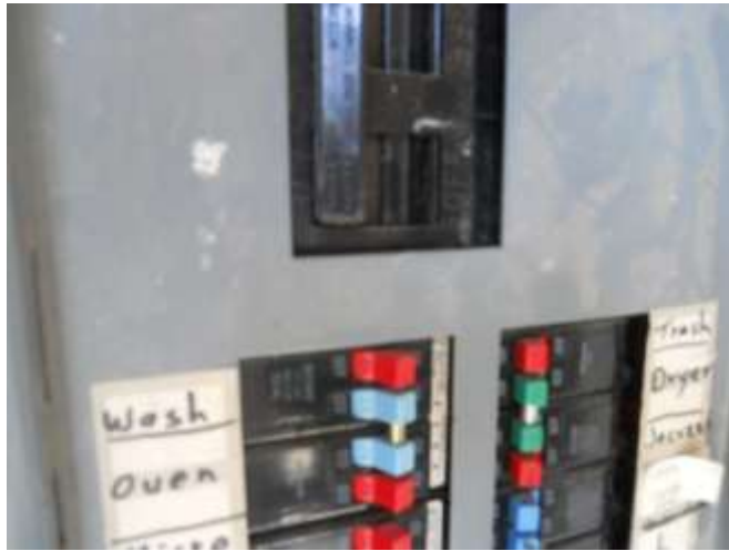
Service panel cover does not fit properly on panel
