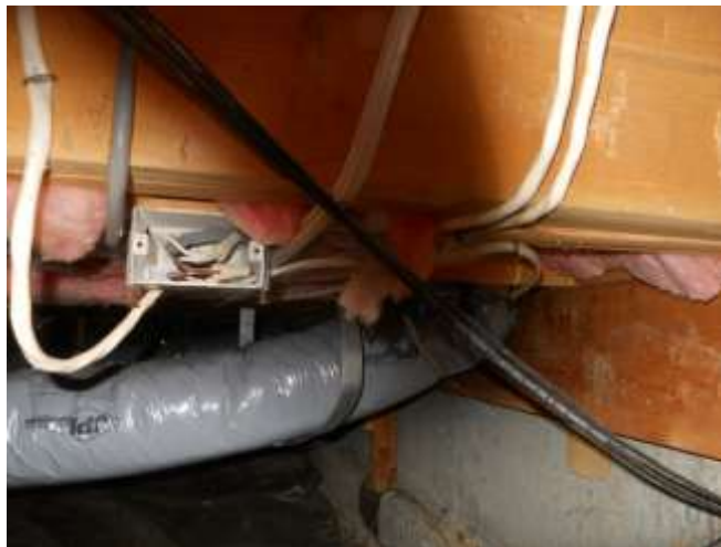
Junction boxes should have cover-plates
