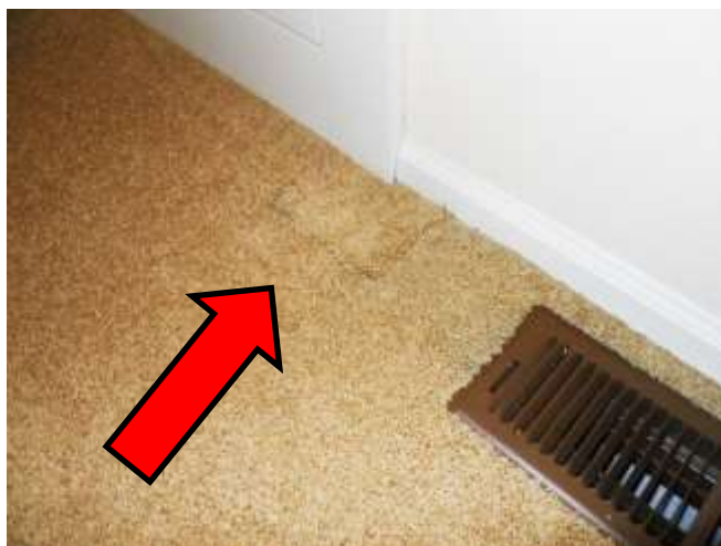
Cut in carpeting
