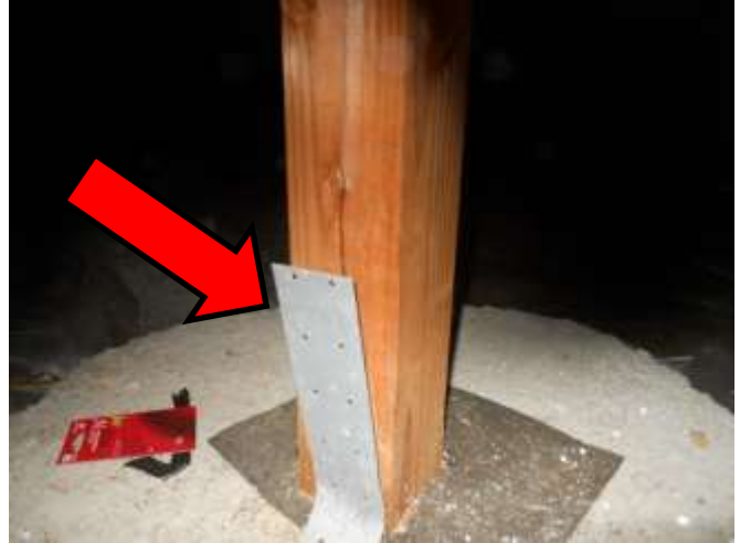
Post strap not secured
