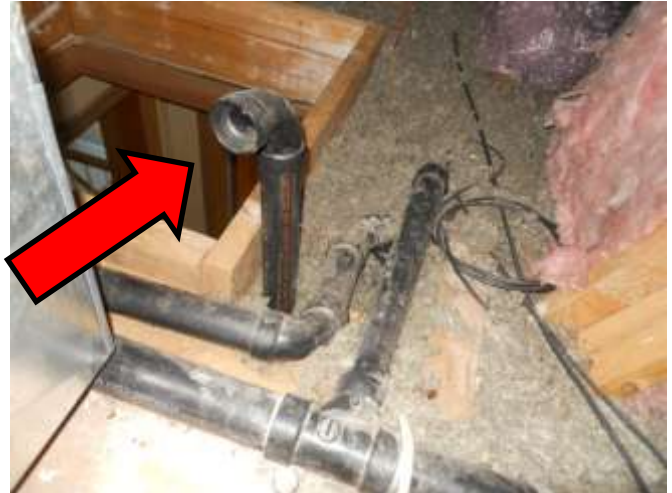
Open plumbing vent stack
