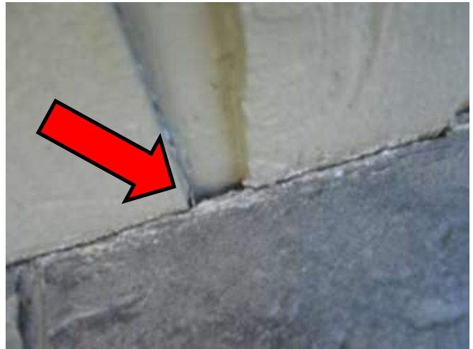
Gaps at siding can lead to trapped moisture
