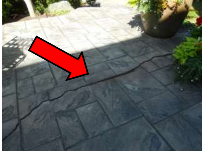
Crack with vertical displacement at stamped concrete patio
