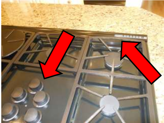
Ventilation control pad is melted Loose burner control indicator
