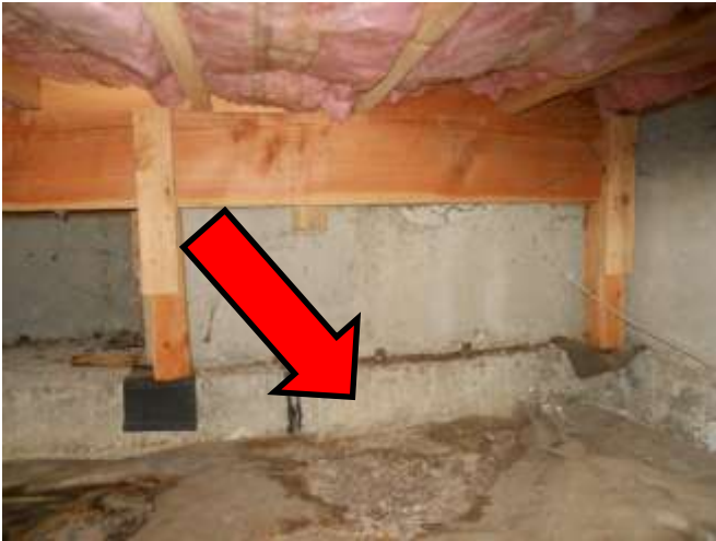
Puddle below Living Room
