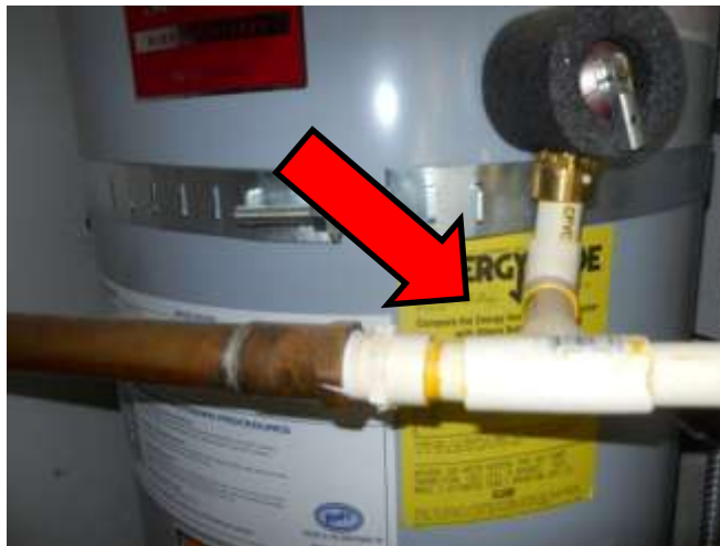
TMP drain lines are tied together
