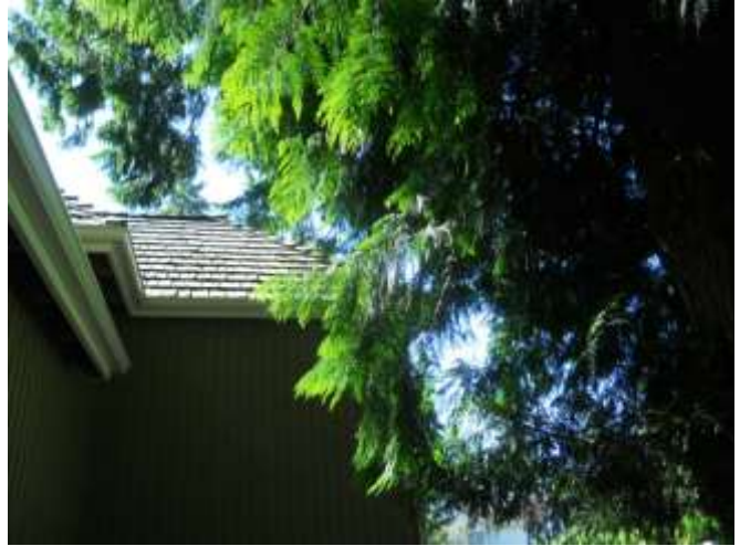
Vegetation in contact with house (typical)
