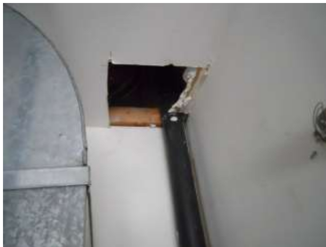
Hole cut in garage ceiling
