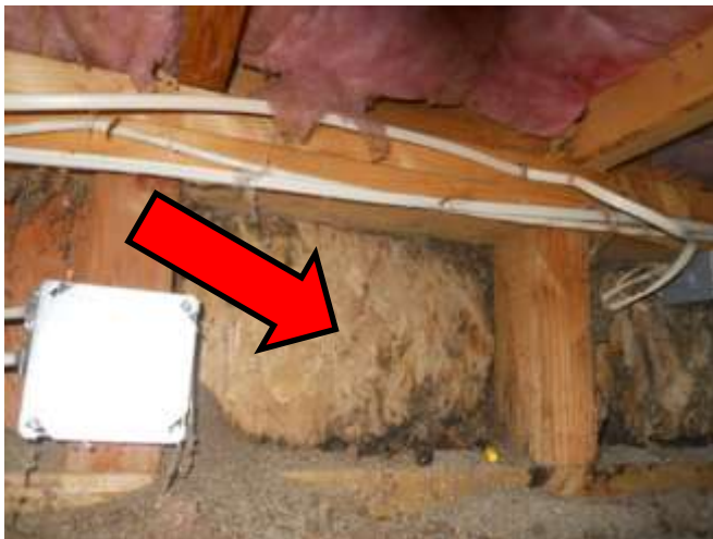
Wood rot near patio door
