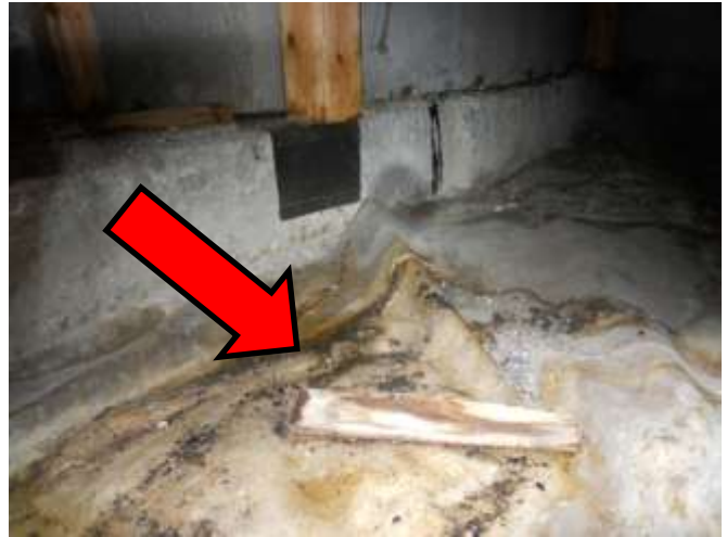
Moisture stains on vapor barrier
