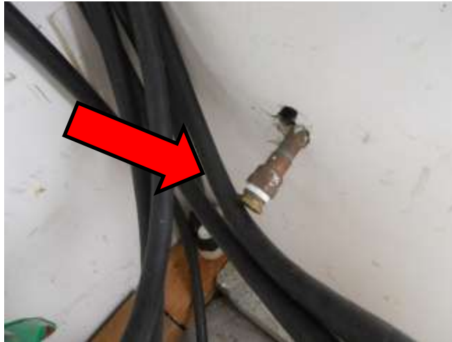
Pipe is capped near electrical panel area
