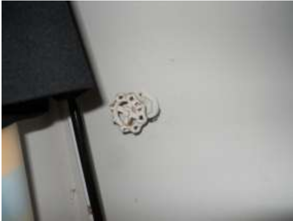
Domestic Water Shut off
