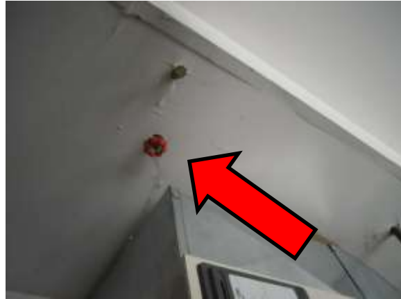
Valve at garage ceiling
