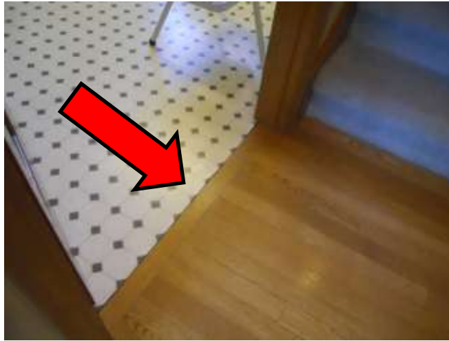
Loose vinyl flooring
