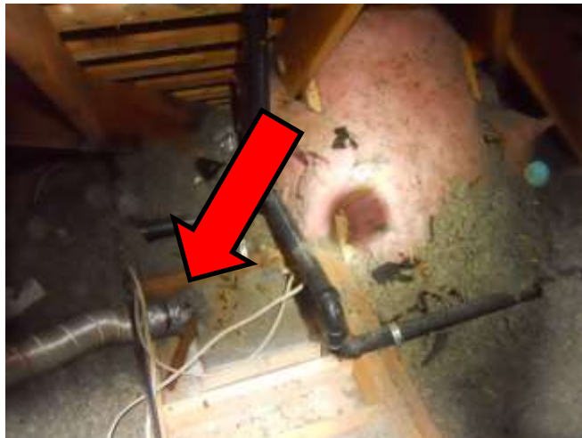
Air is blowing into attic from main bedroom suite fan
