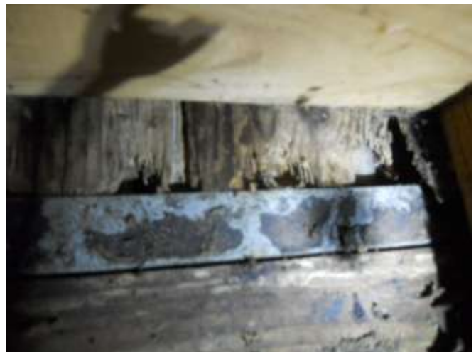
Wood rot near patio door Visible boards are siding
