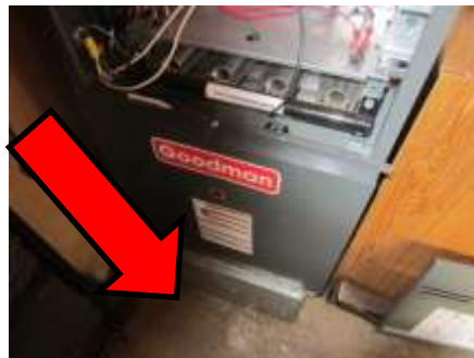
Furnace filter location
