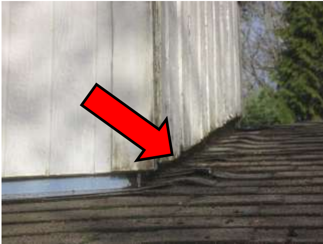
Flashing does not lay flat of roof
