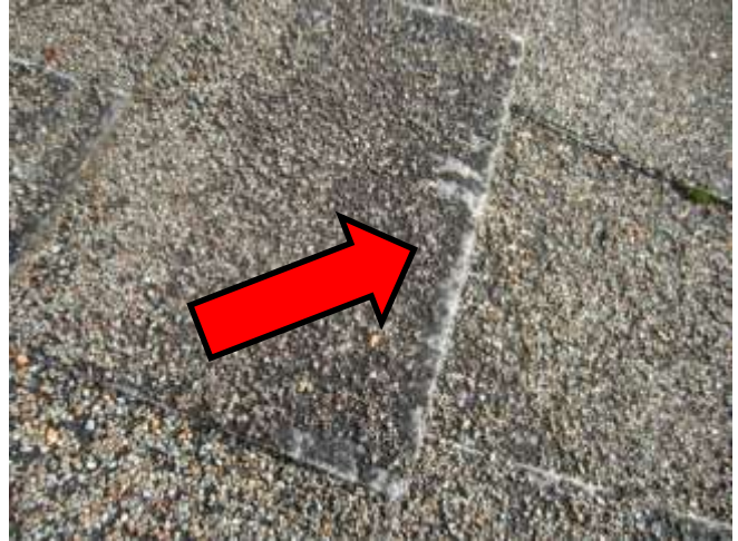
Fibers visible at shingle (typical)
