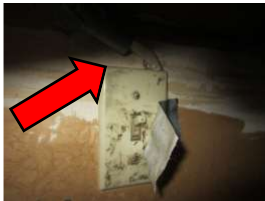
Surface wires in the garage
