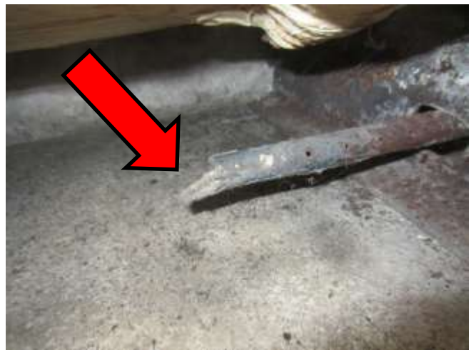
End of log lighter is gone (rusted)
