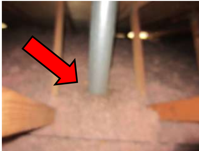
Insulation should not be in contact with the flue
