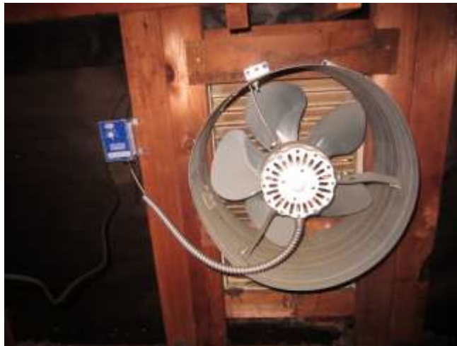
Attic ventilation system
