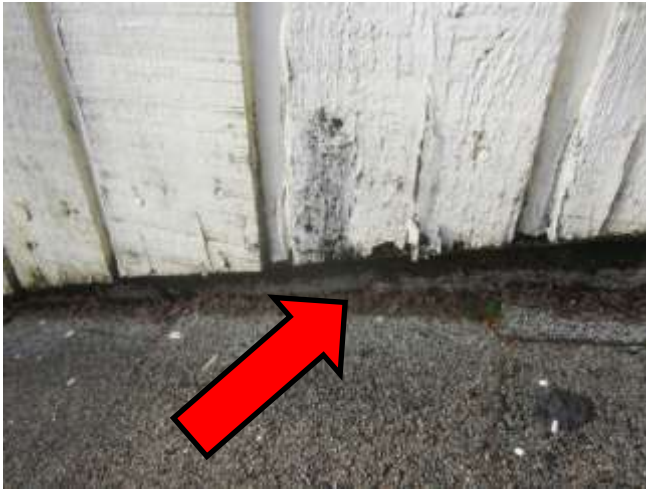
Minor wood rot at chimney siding
