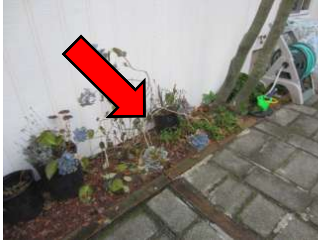
Siding in contact with the ground
