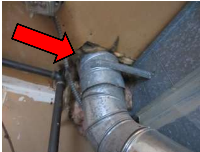
Furnace flue in contact with insulation and drywall
