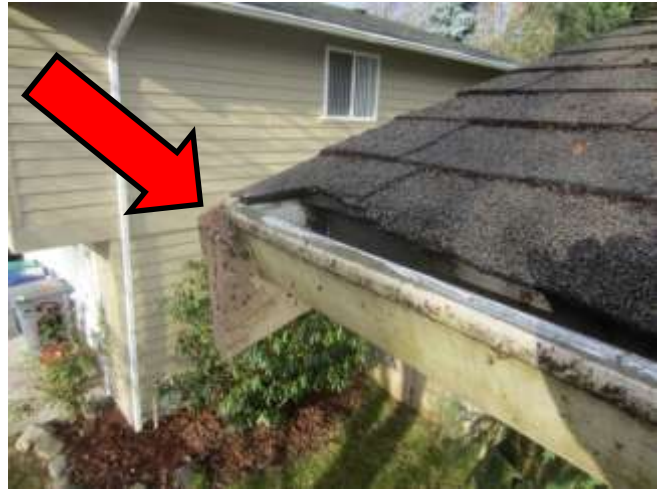
Minor wood rot at fascia boards (tails)
