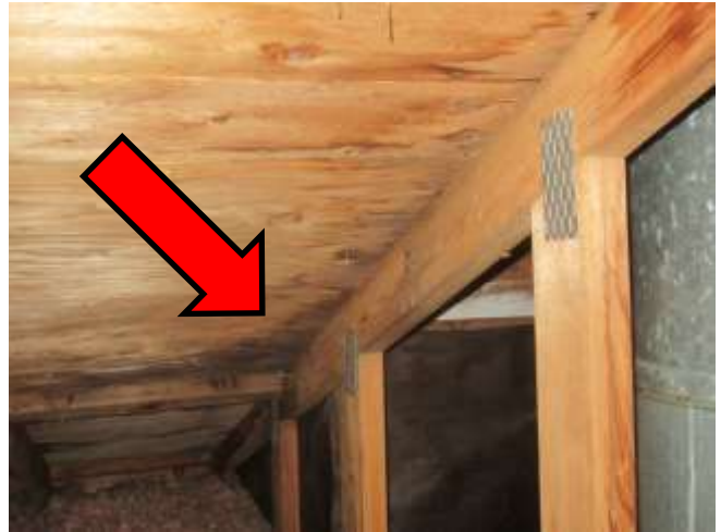
Area below image to left (arrow points to moisture stains)
