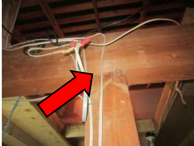
Recommend additional post to beam connection
