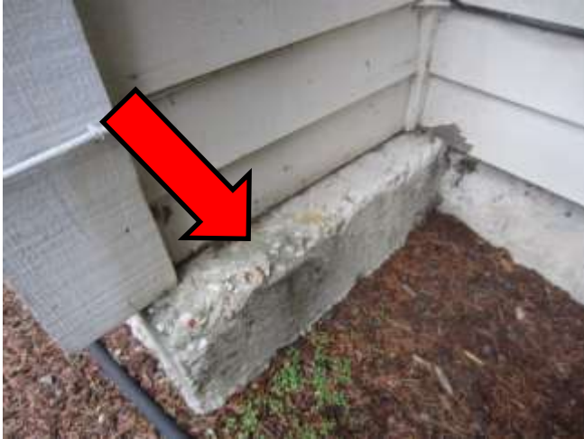
Flashing missing at concrete foundation
