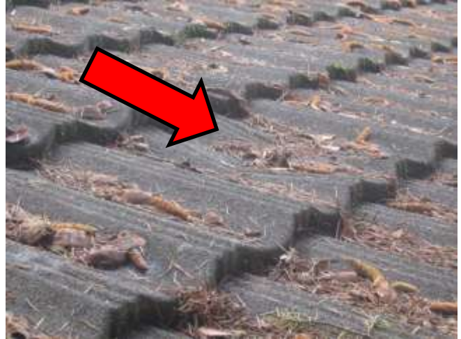
Crushed roofing (typical)
