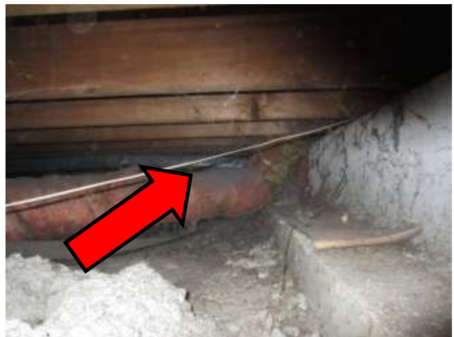
Lint at crawlspace
