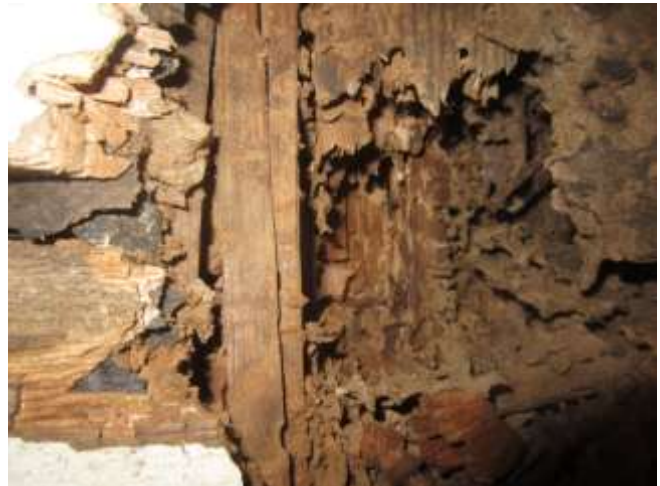
Moisture ant damage
