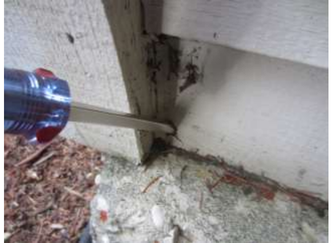
Wood rot (see image to left)
