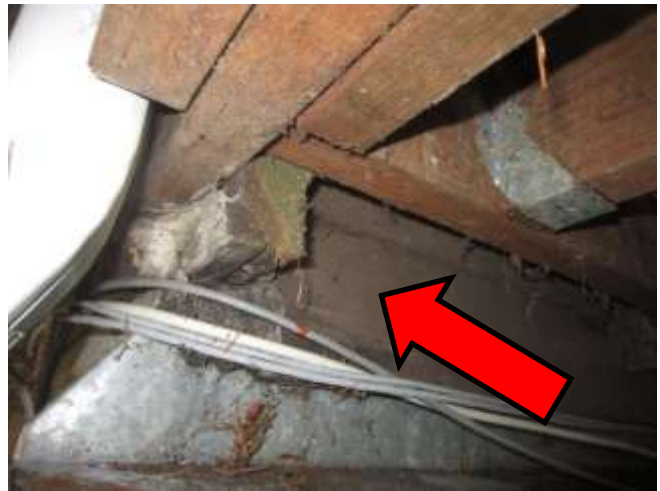
Area above moisture ant damage
