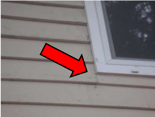
Caulking not complete at Master Bathroom
