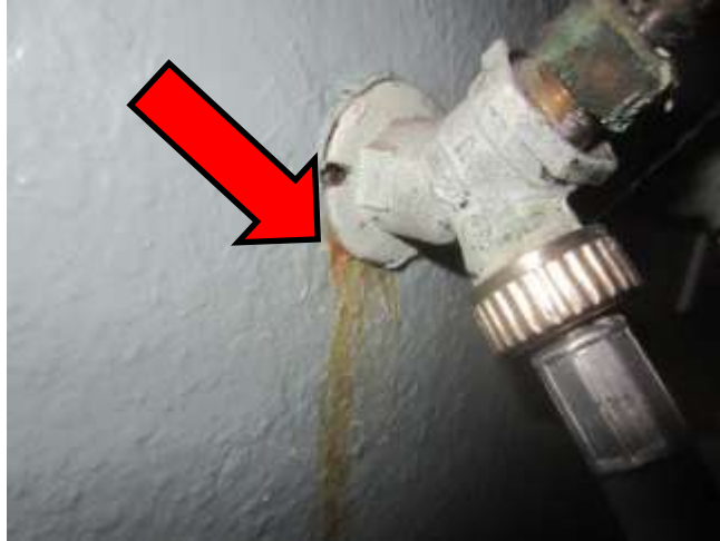
Evidence of moisture leak from washer supply line
