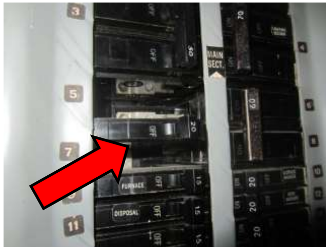
Missing knockout covers
