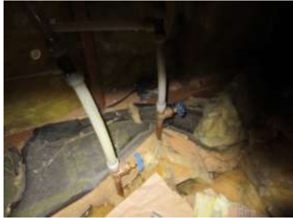
Plastic domestic water pipes
