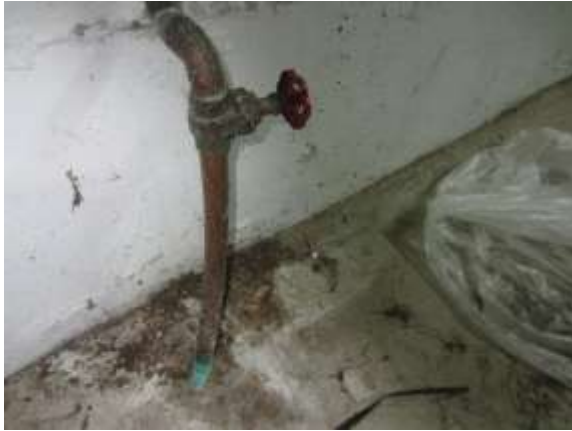
Domestic Water Shut off
