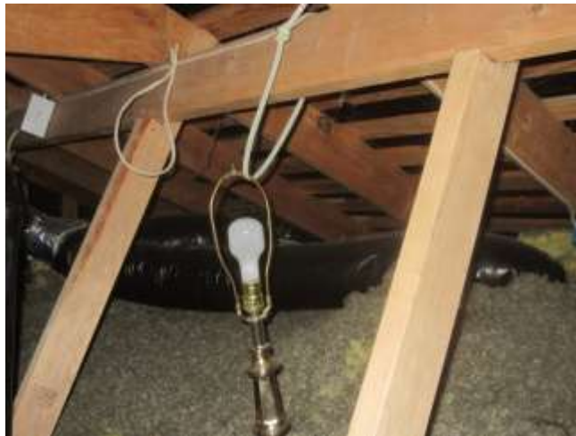
Improper attic light
