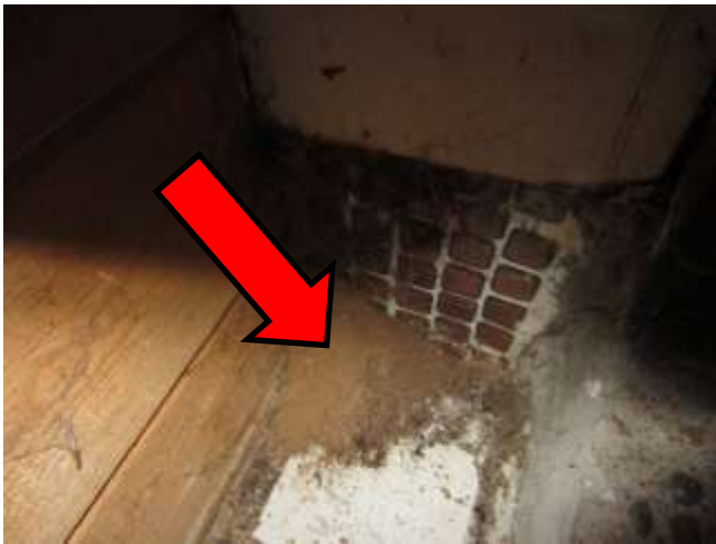
Moisture ant damage
