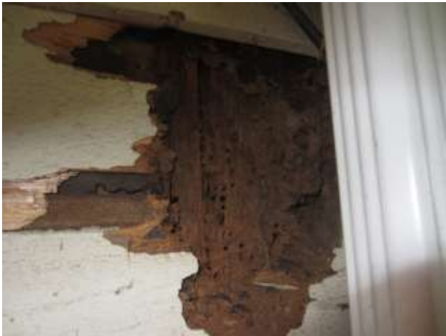
Moisture ant damage
