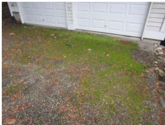
Slip hazard at driveway due to moss build up
