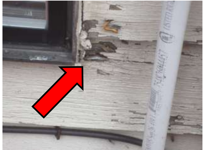
Moisture damage at Siding
