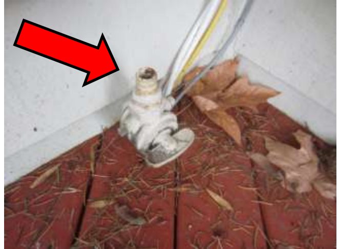
Open gas valve at deck
