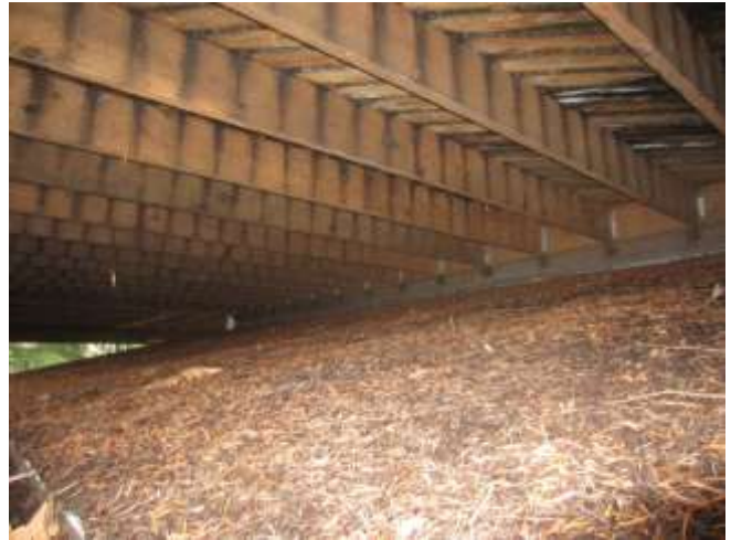
Debris on hot tub area extension roof
