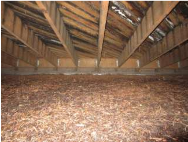
Debris on hot tub area extension roof
