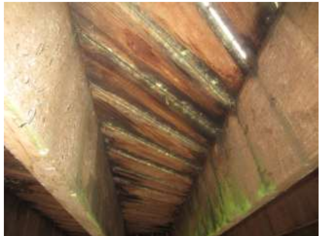
Minor wood rot at decking (typical)
