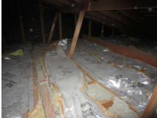
Vapor barrier on cold side of insulation above blown in insulation. This configuration can lead to condensation
