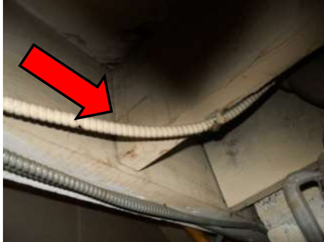
Joist hangers should be installed
