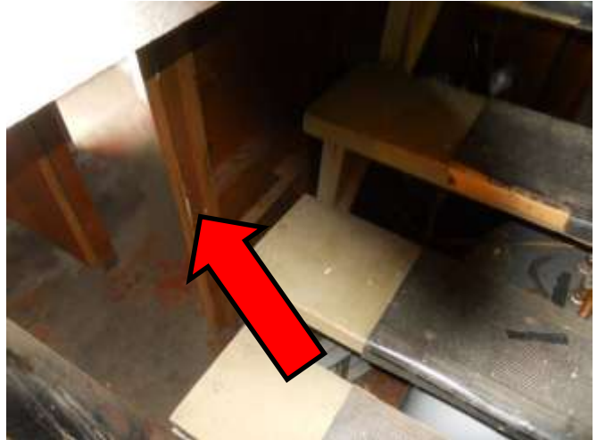
Barricade missing entirely
