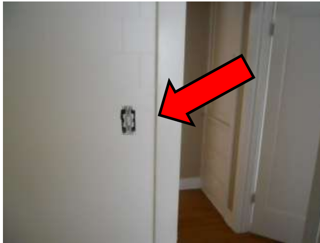
Light switch in shower area
