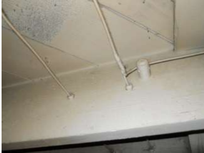
Knob and tube wiring in basement
