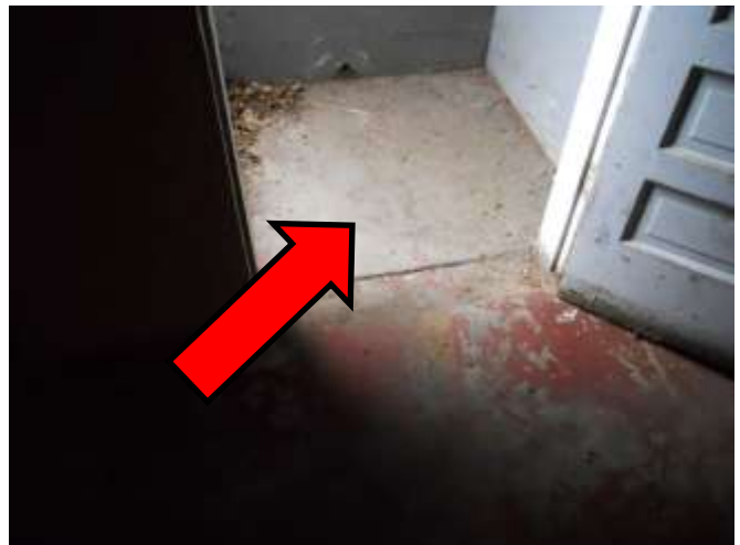
Floor drain missing from side stairwell
