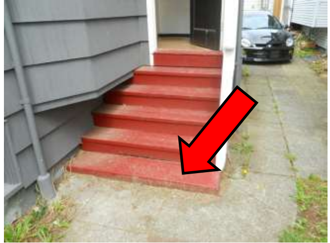
Trip hazard at stairs
