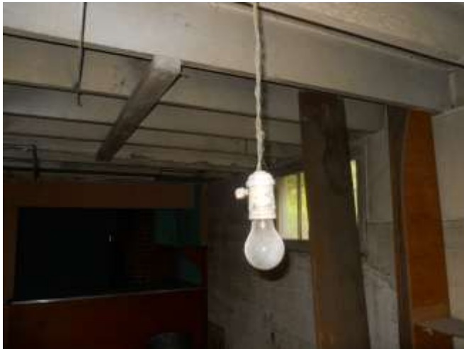
Existing light fixture
