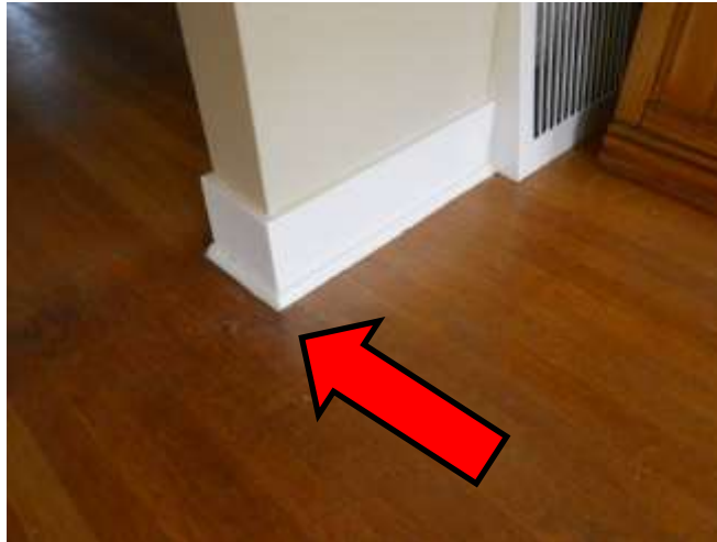
Structural sag at Living room
