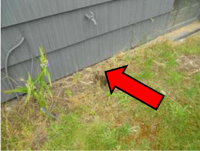
Exterior grade is in contact with siding
