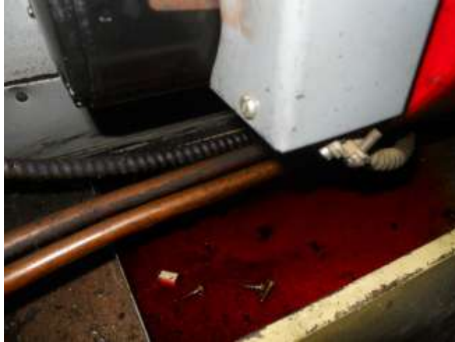
Oil leak at furnace
