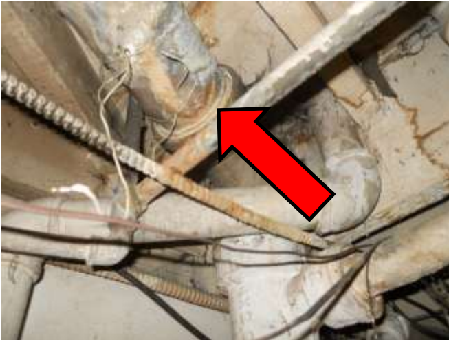
Cracked waste line
