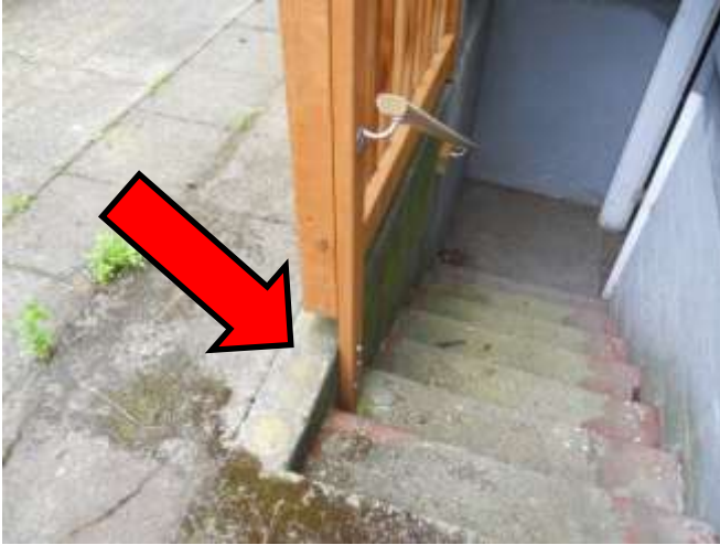
Barricade and handrail should extend to top
