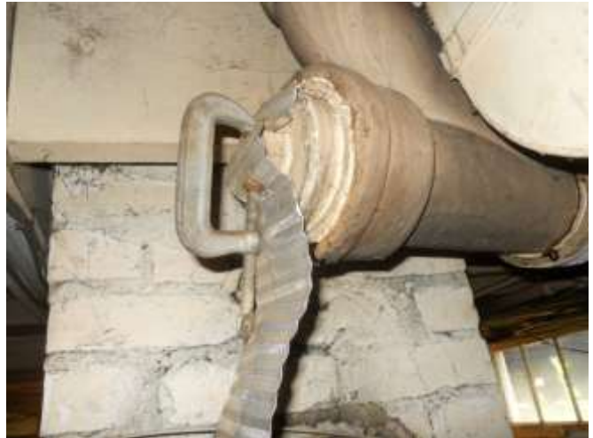
C clamp on waste line
