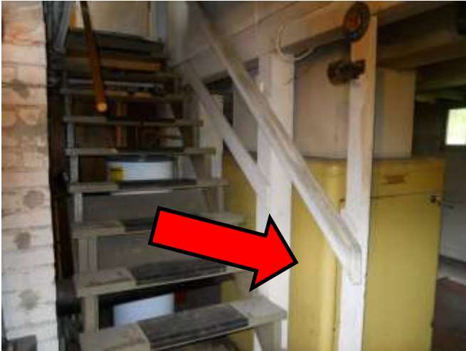
Barricade safety hazard
