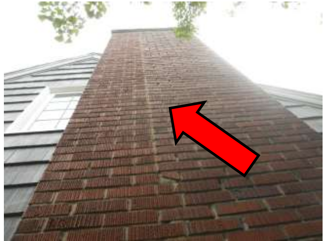
Fireplace appears to have been modified since original construction
