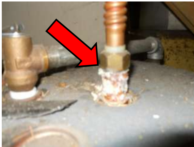
Corrosion at water connection
