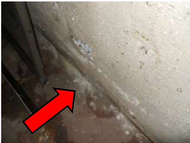
Evidenec of moisture intrusion at N.W. wall
