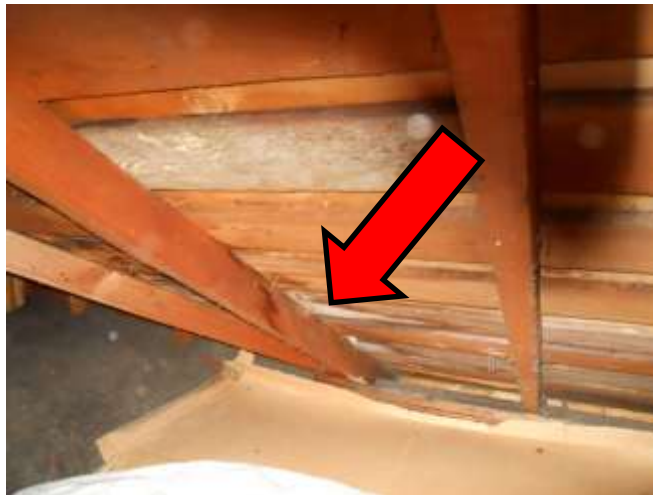
Area of possible moisture intrusion
