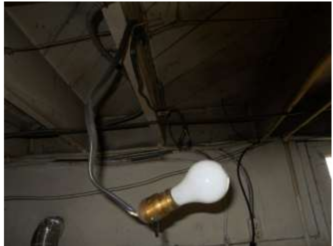
Existing light fixture
