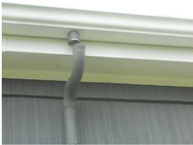
Downspout not connected
