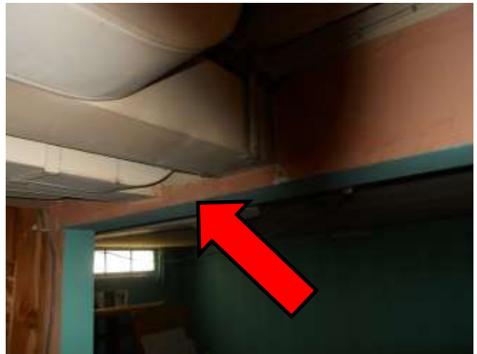
Beam has been over notched Floor is sagging above
