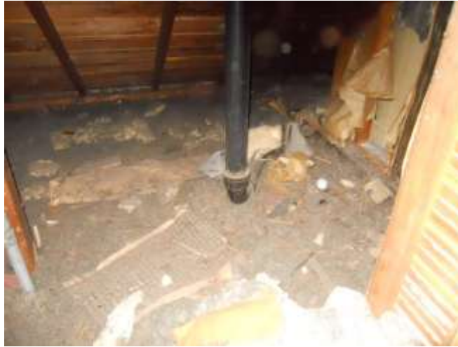
Debris should be cleaned from attic area
