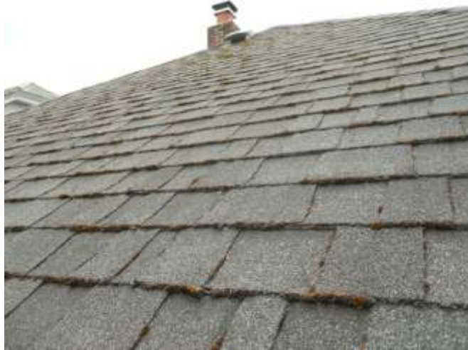
Moss buildup at roof (typical)
