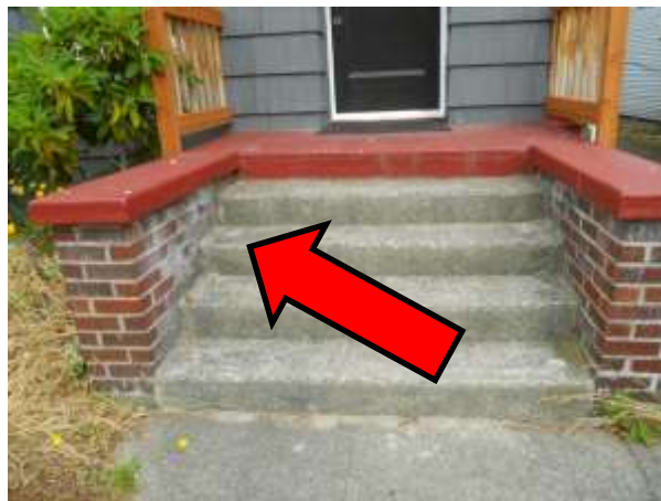
Graspable handrail not installed
