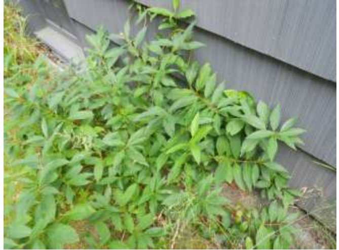
Vegetation in contact with siding
