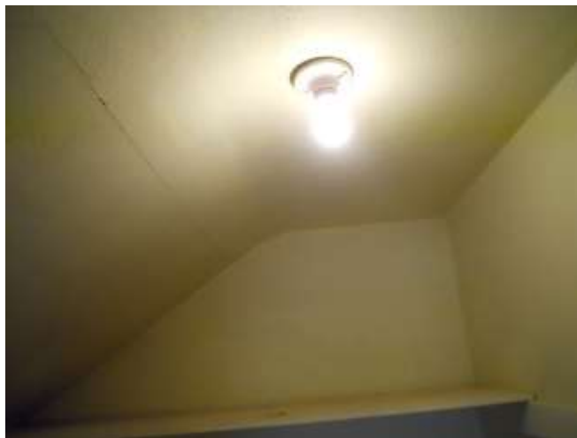
Fire hazard at exposed bulb light fixtures
