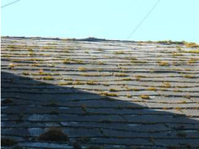
Moss build up at roof
