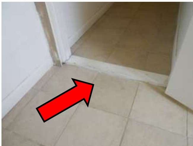
Trip hazard at entryway to room
