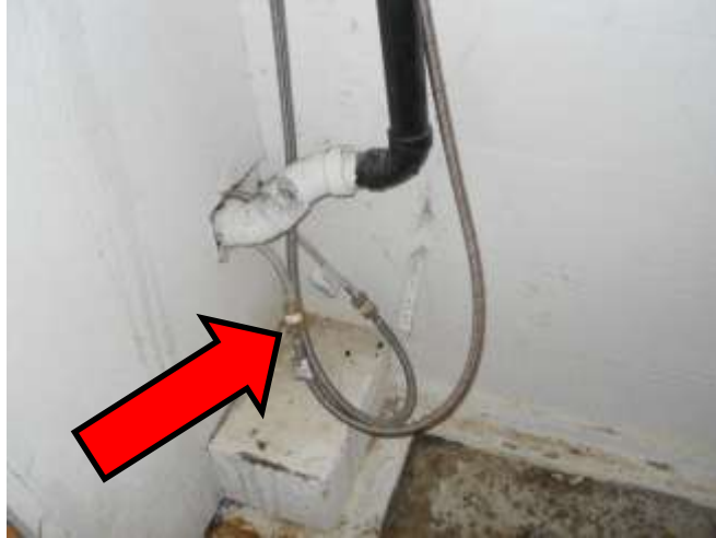
Improper extension of water supply lines to sink
