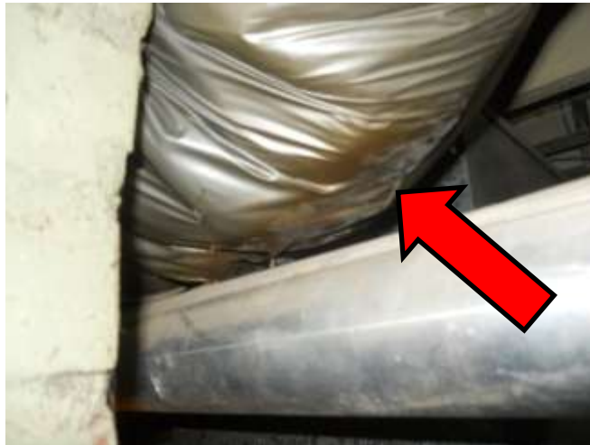
Insulation cover of heat duct is melting
