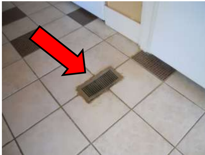
Trip hazard at heat register in middle of room
