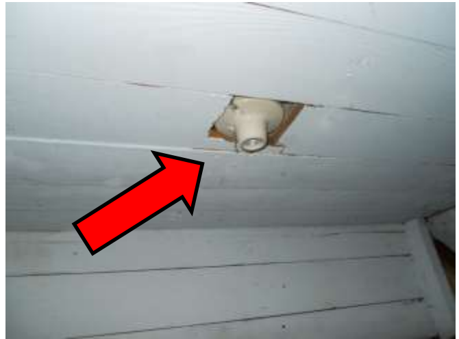
Exposed light bulb fixtures are a fire hazard Items could get into contact with hot light bulbs
