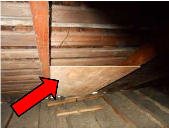
Evidence of prior leak Board is placed to divert rainwater
