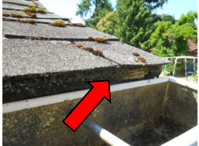
Sheathing deterioration at edged
