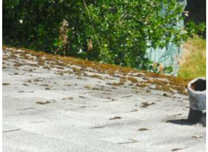
Moss build up at roof
