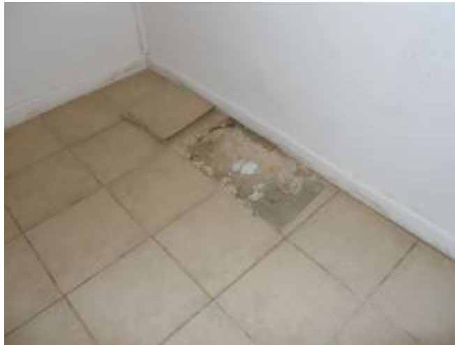
Loose tiles at mechanical room due to moisture
