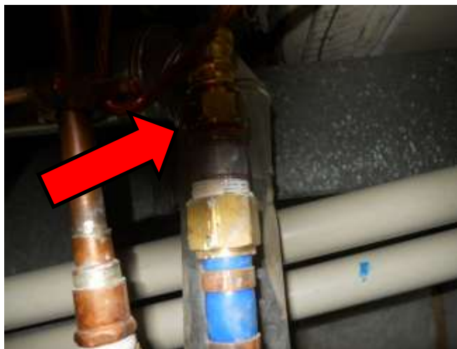
Corrosion at water pipe connection
