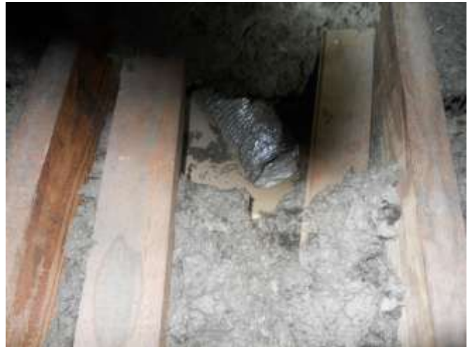
Vent should be extended to the exterior
