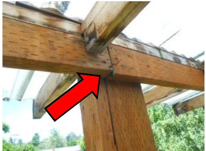
Provide proper connection from deck cover supports to posts (metal strap)
