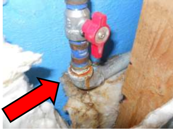
Leak at domestic Water Shut off
