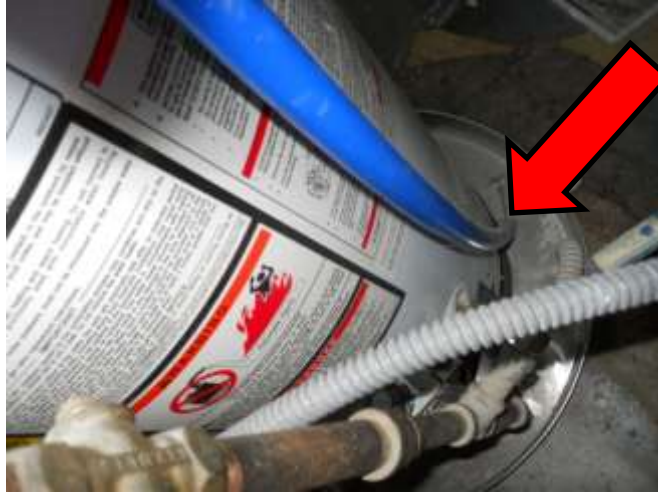
TMP drain line should not be blocked
