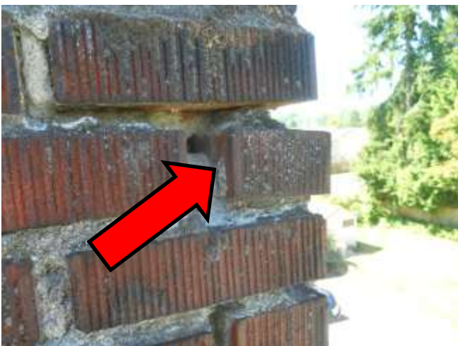
Deterioration of mortar
