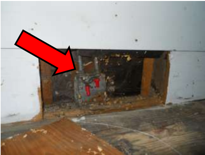
Cover plate missing at junction box
