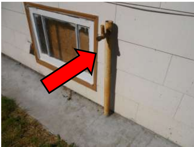
Evidence of abandoned oil tank
