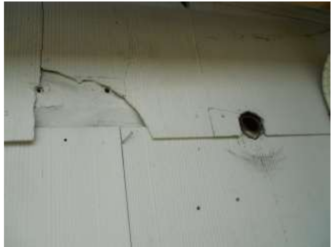
Damaged siding (typical)
