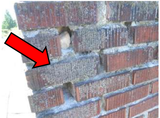
Deterioration of mortar
