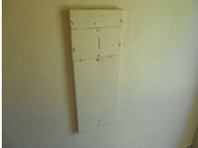
Assumed original electrical panel at floor 1 hallway
