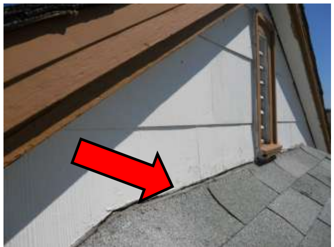
Roof to wall flashing not installed
