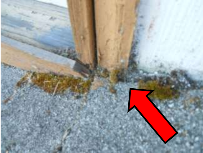
Flashing not installed at window above rear entry
