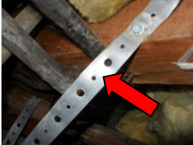
Edge of Metal strap in contact with electrical wire
