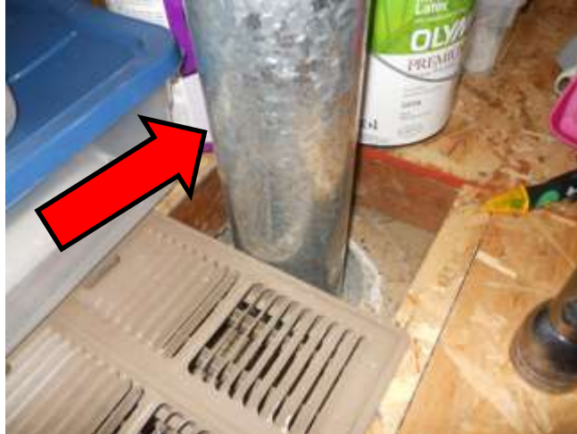
Furnace flue should have shield to prevent combustibles from coming within 1”
