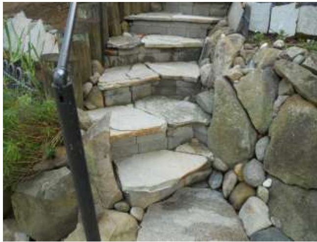
Uneven stairs to rear yard
