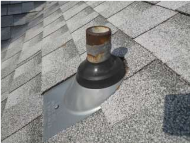
Plumbing vent stack should extend 6" + above roof
