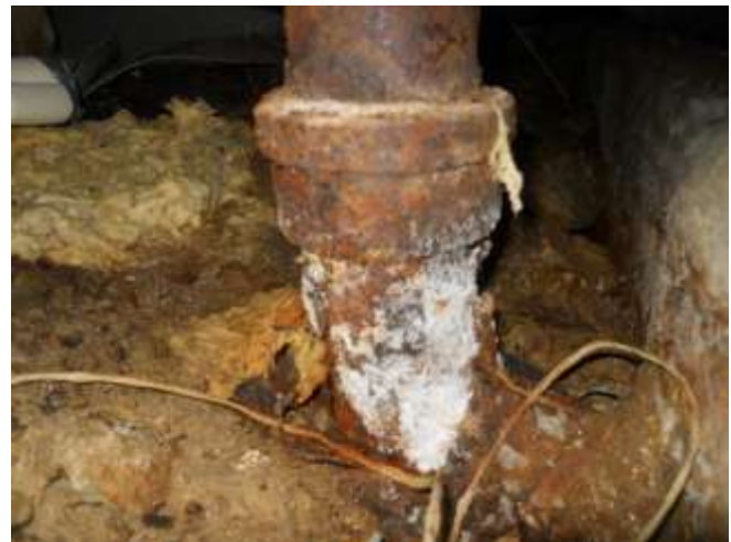
Deterioration of sanitary sewer pipe View from South
