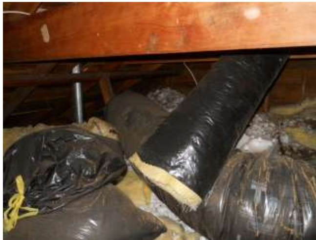
Debris in attic
