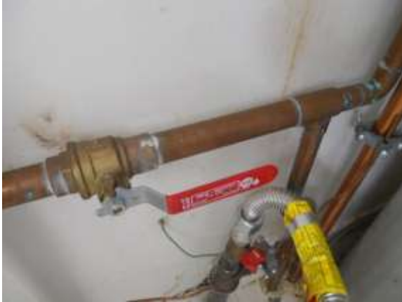
Domestic Water Shut off
