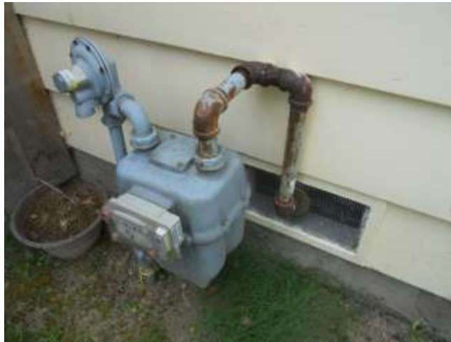
Current code would not allow a gas meter to be located within 3' of a foundation vent
