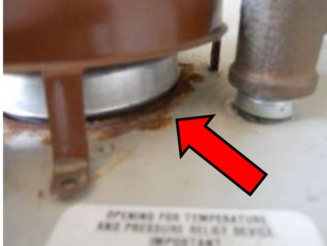
Evidence of inadequate draft at the water heater flue
