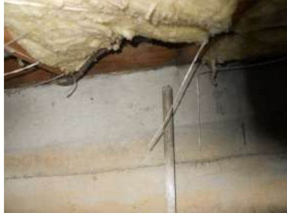
Abandoned galvanized supply line
