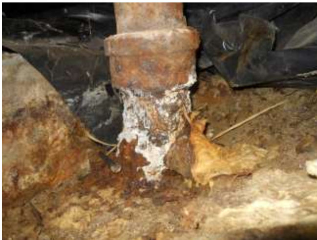
Deterioration of sanitary sewer pipe View from North
