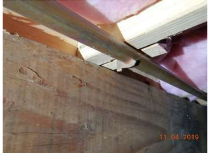
Domestic water distribution pipes
