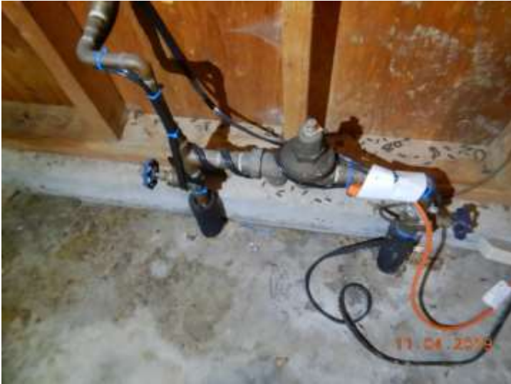
Domestic water shut off
