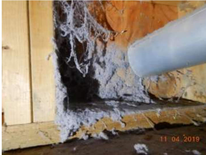
Evidence of lint leakage
