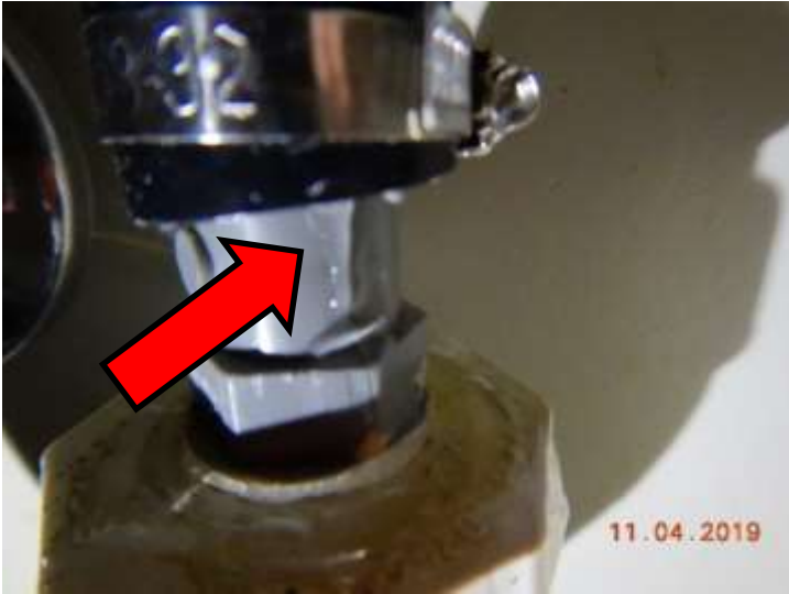
Leakage from the dishwasher drain
