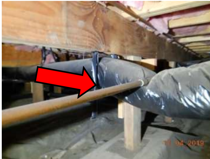
Pipe not secured to the framing
