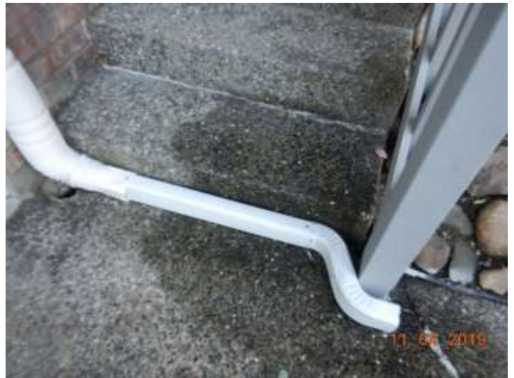
Evidence of water discharge onto the walkway and driveway
