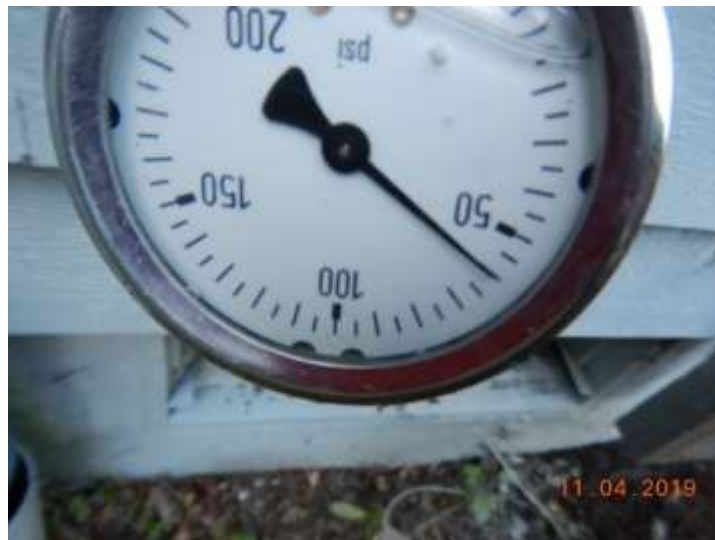
Water pressure is adequate and not excessive
