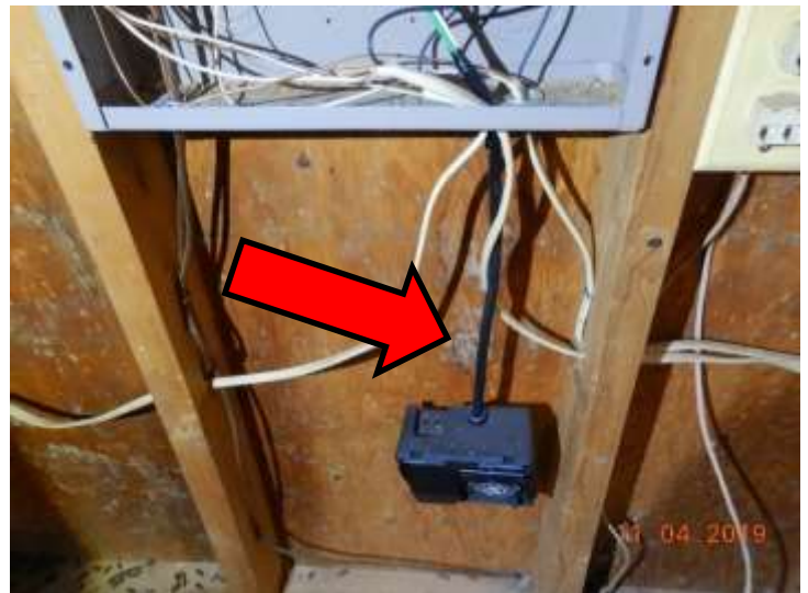
Homeowner added wiring/ outlet
