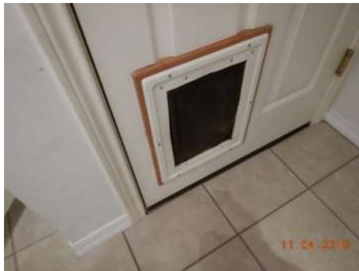
Pet door cut into the door to the house
