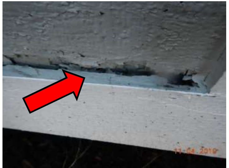
Evidence of wood rot
