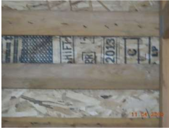
The roof appears to have been installed in 2013 based on the date stamp of the roof sheathing
