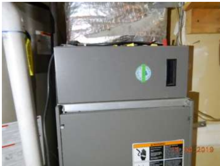
Furnace filter location
