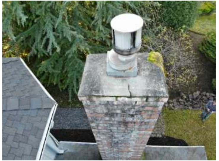
Chimney. A minor crack is visible at the cap
