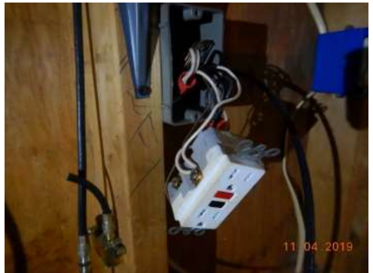
Unsecured GFCI outlet
