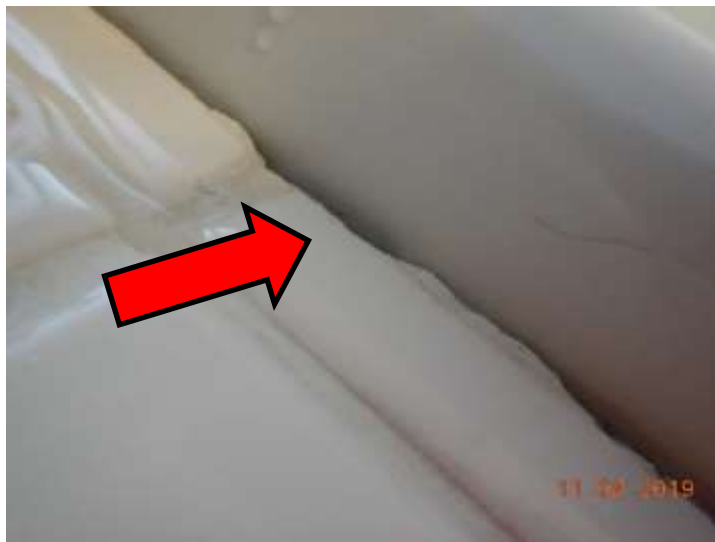
Gaps surrounding the bathtub
