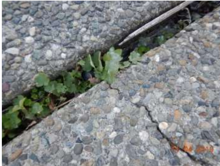
Cracks at the driveway, rotted out expansion joints
