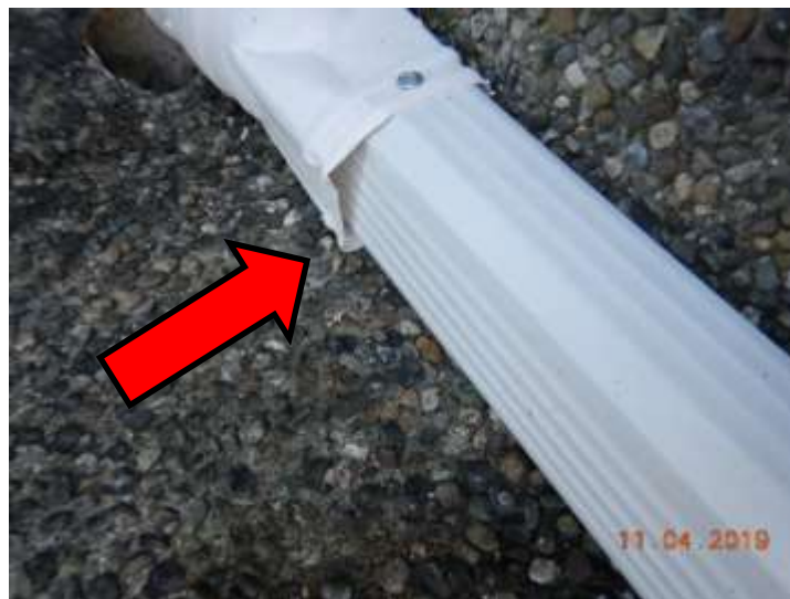
The connection of the extension is installed backwards which will allow leakage
