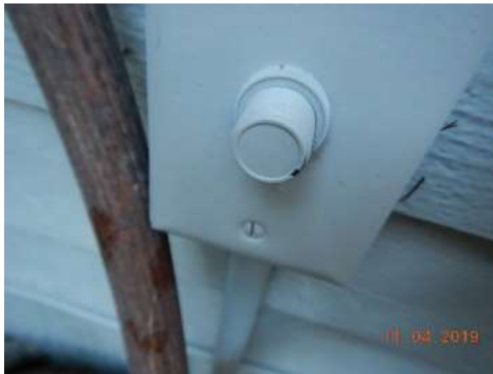
Painted photocell sensor
