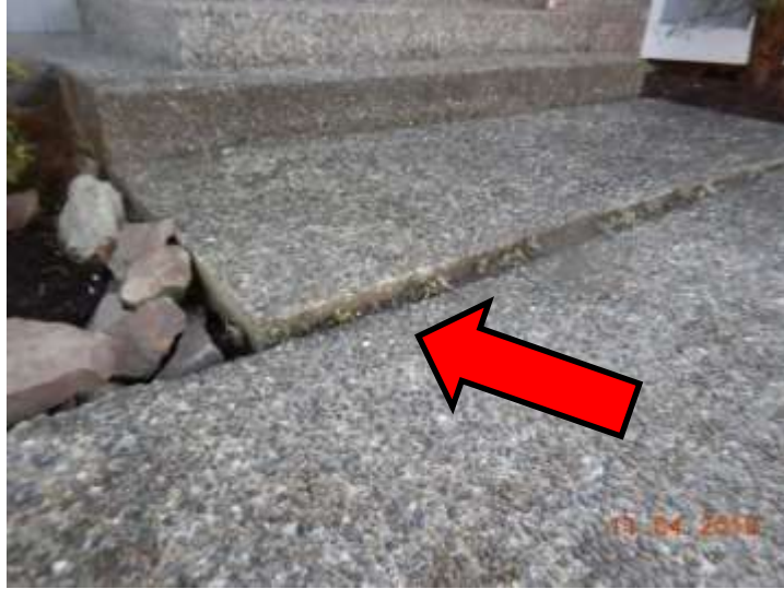
Trip hazard at the vertical displacement
