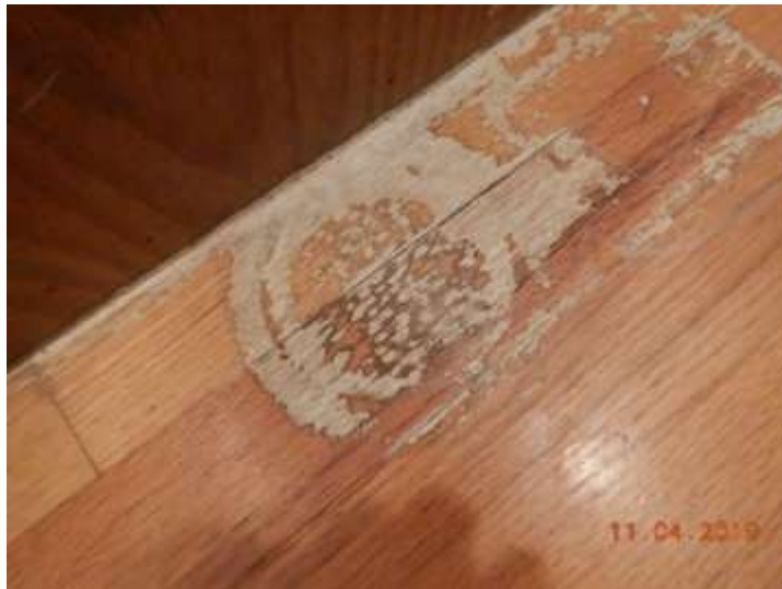
Prior surface damage to the hardwood flooring. Appears to be from a prior pet dish
