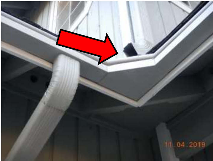
The upper downspout will overshoot the lower gutter during strong rain events
