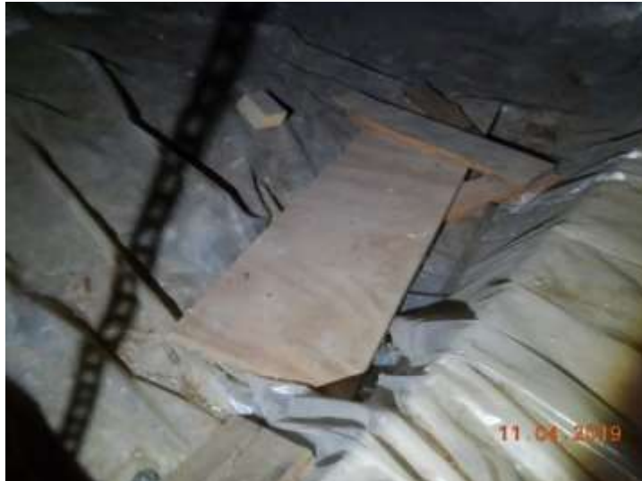
Debris in the crawlspace (typ)
