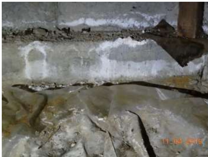
The white is evidence of high moisture, however no moisture intrusion was noted
