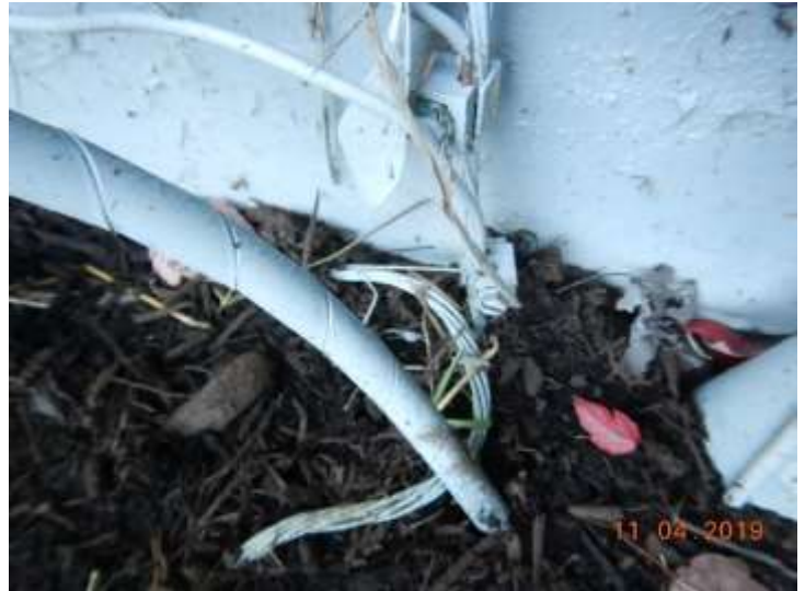
Electrical system grounding
