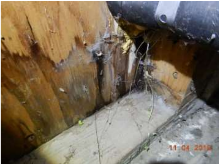
Evidence of wood rot
