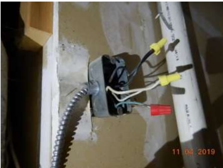
Open electrical wires
