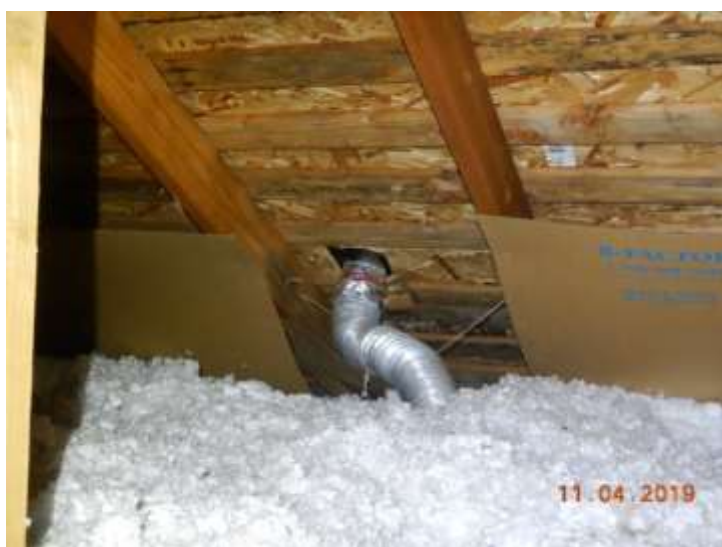
Bathroom ventilation duct
