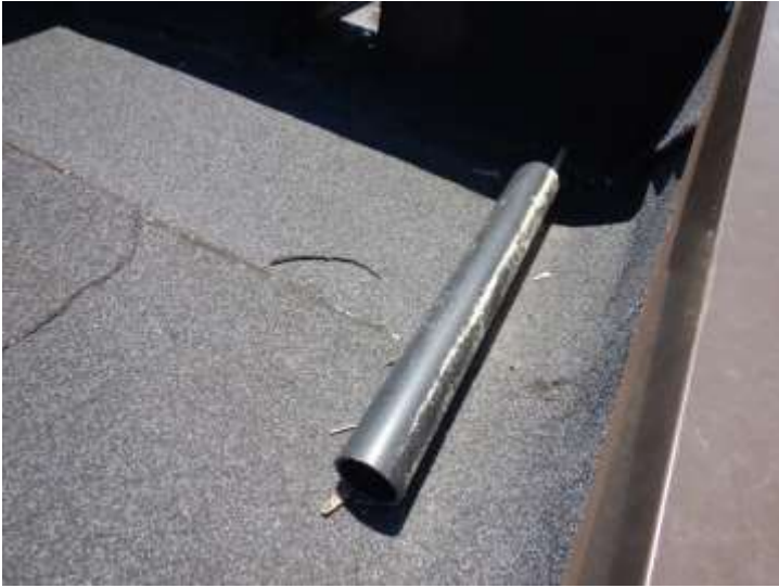
Debris on the roof
