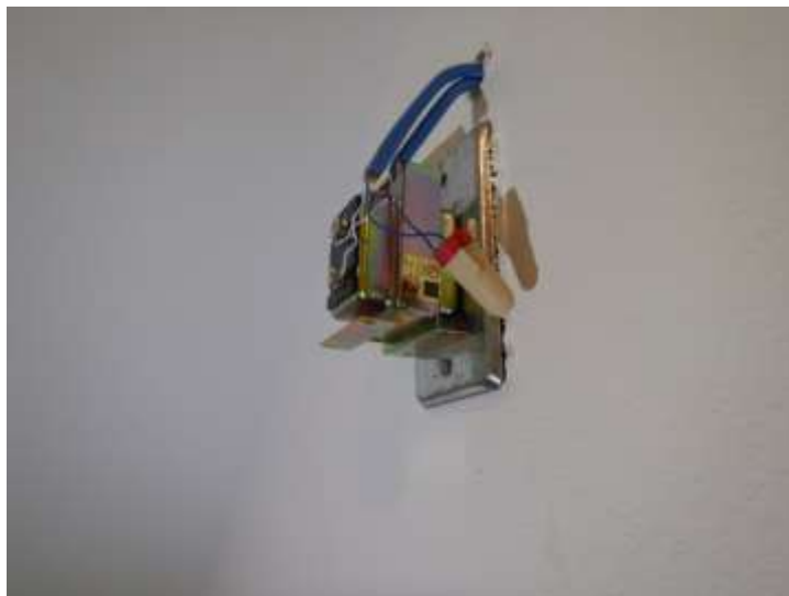
The doorbell transformer is located in the closet
