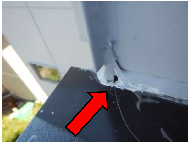
Gap at the wall cap caulking
