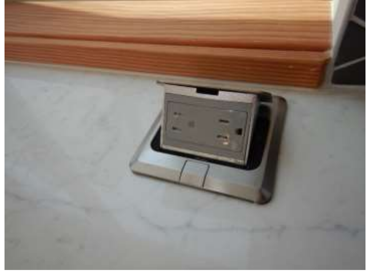
Countertop electrical outlet
