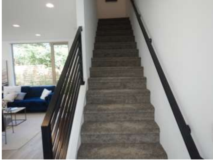
There is a slight West-East lean to the stairs
