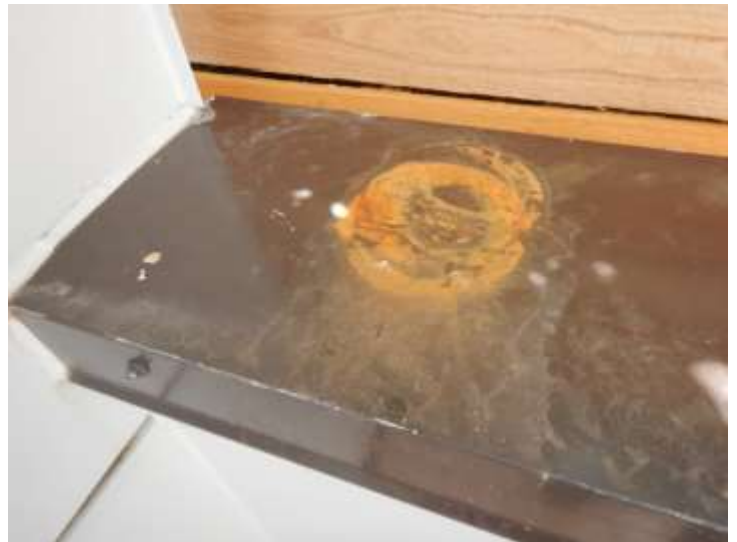
Rust stains at the wall cap
