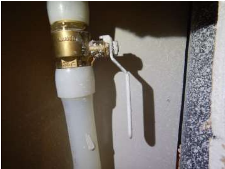
Domestic water shut off
