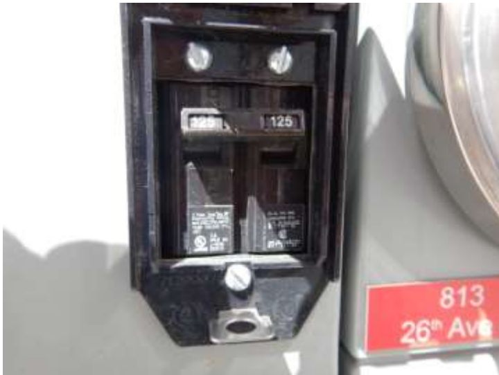
Electrical system disconnect
