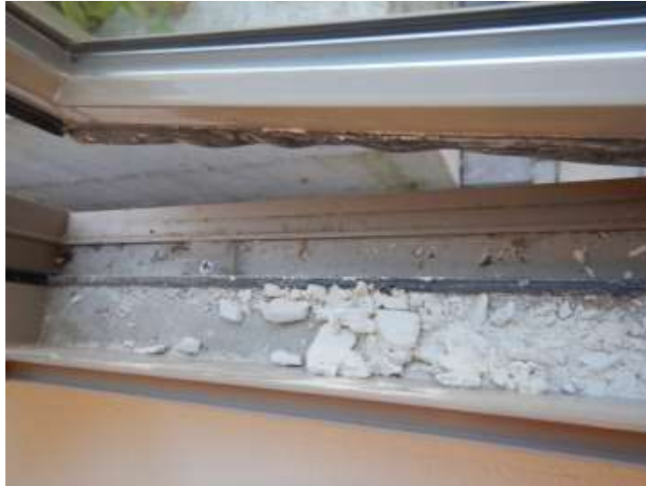
Debris in a window track
