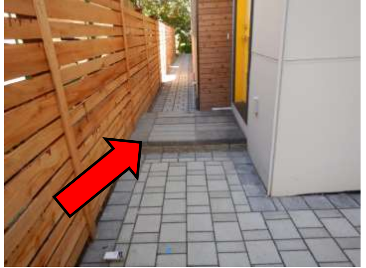
Trip hazard, no common area walkway illumination is provided
