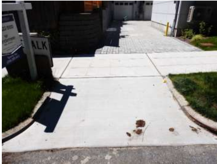
The driveway apron is not in alignment with the driveway
