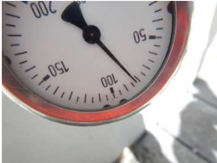
Water pressure is adequate and not excessive
