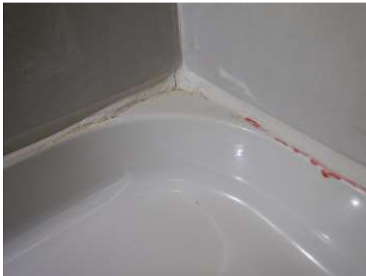
Debris/ marks at the tub surround
