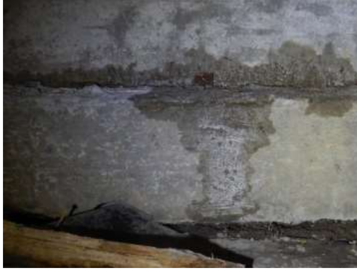
Evidence of moisture intrusion
