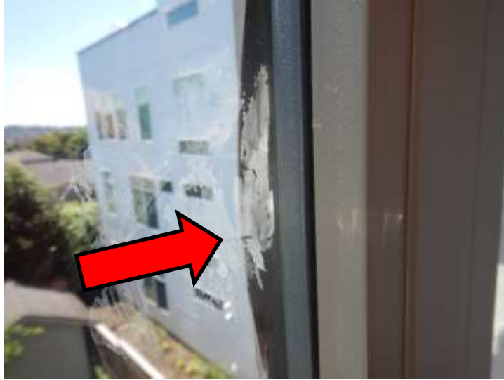
Loose glass stop
