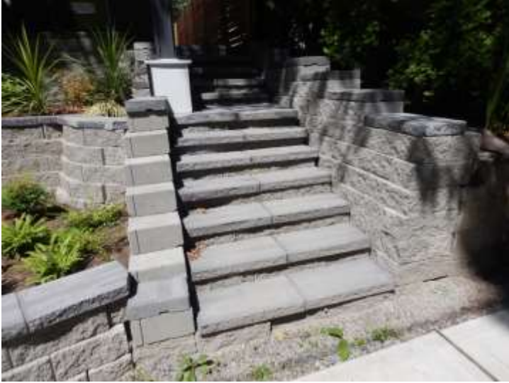
A graspable handrail is not installed
