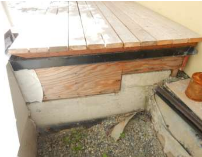
Missing barricade - exposed non weather rated wood
