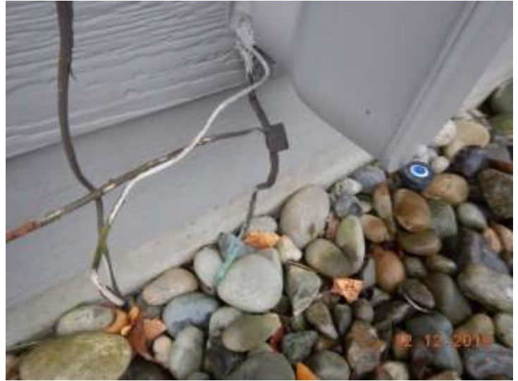
Electrical system grounding
