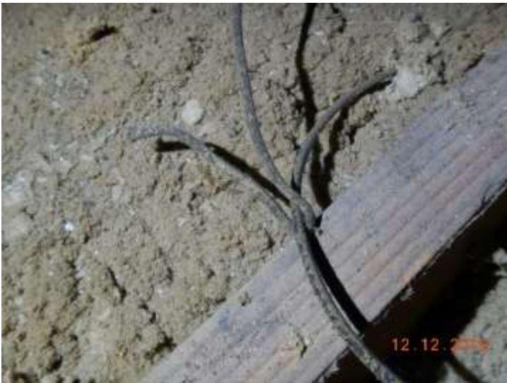
Loose and uncapped wire (live)
