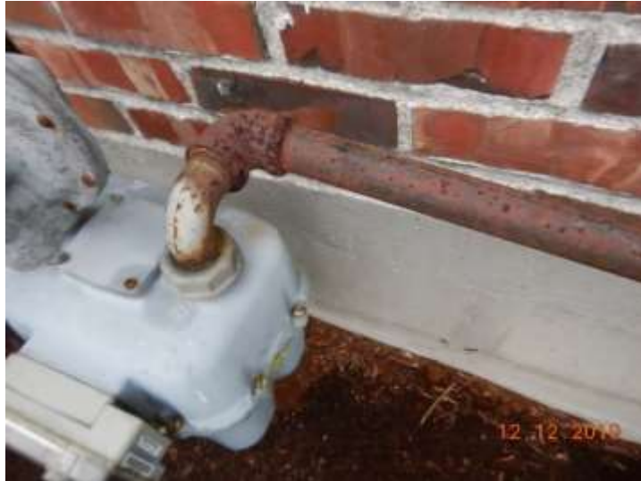
Rusting gas pipes
