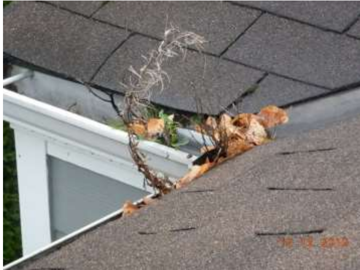
Gutter full of debris and vegetation
