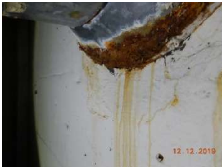
Corrosion of the furnace flue
