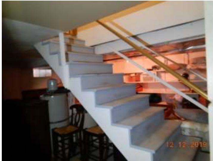
A proper safety barricade is not installed
