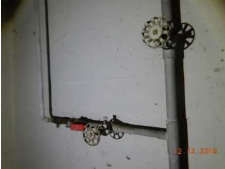
Domestic water shut off
