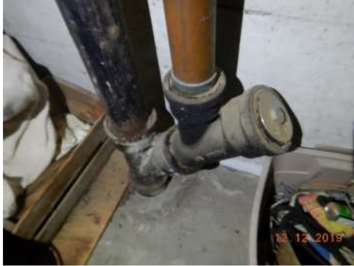
Plumbing waste lines
