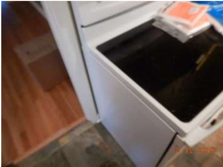
No cabinet or countertop at the side of the range
