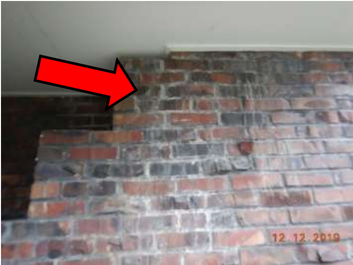
Stains at the entryway wall appear to be older; active leakage was not identified
