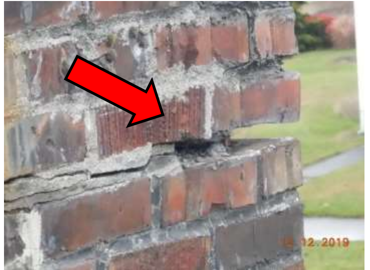
Gaps at the mortar
