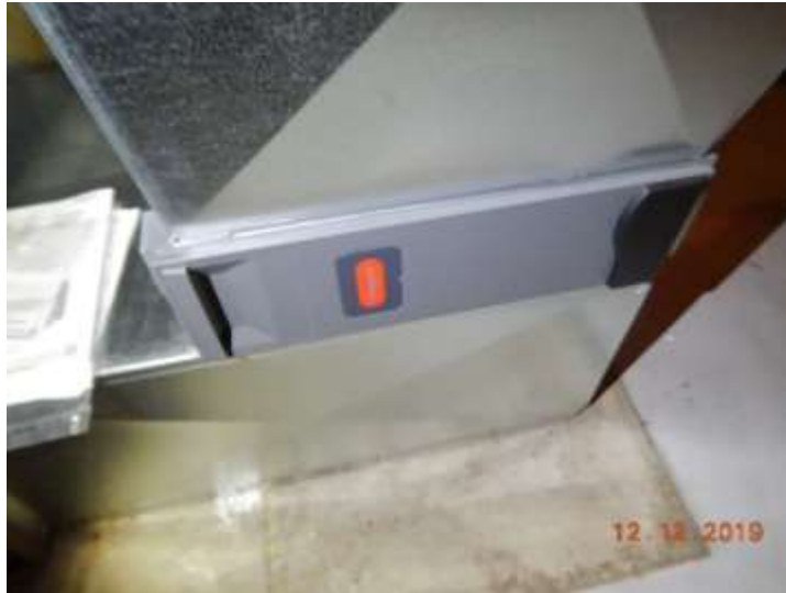
Furnace filter location
