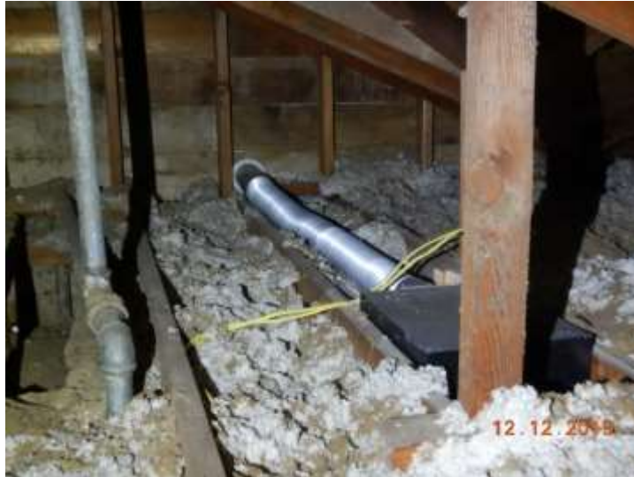
Bathroom ventilation duct
