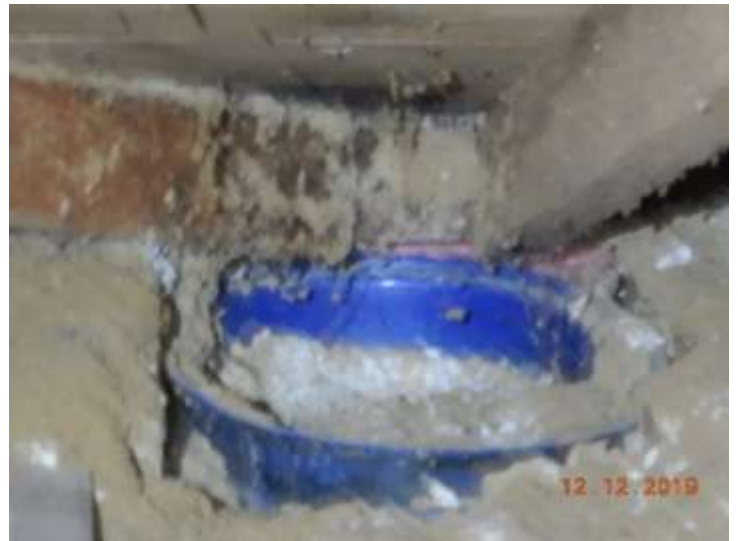
Bucket located in the attic above the North area of the kitchen
