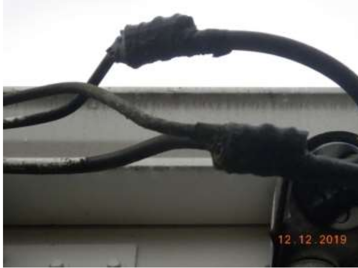
Overhead electrical wires
