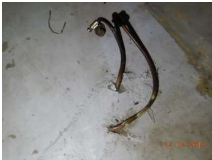
Oil tank lines
