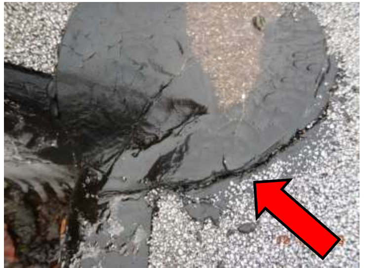
Cracking of the patch
