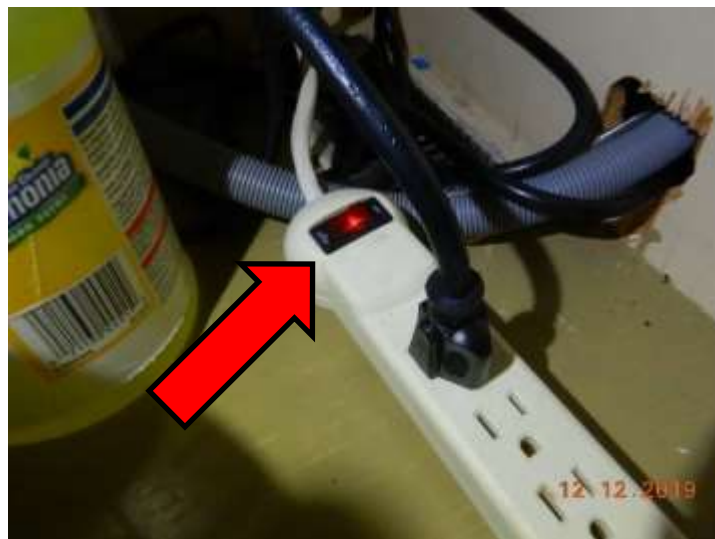
Control switch for the disposal
