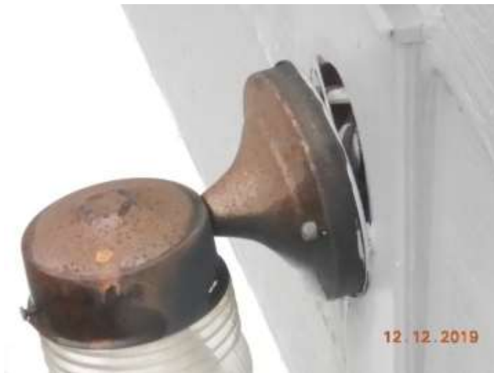
Loose light fixture
