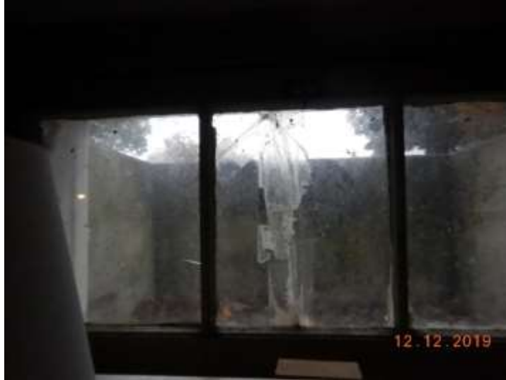
Broken/ taped window
