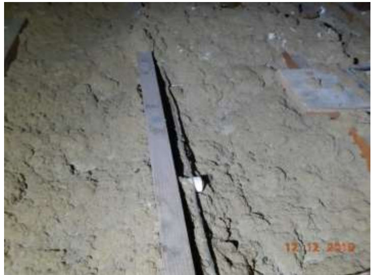
Knob and tube buried in insulation
