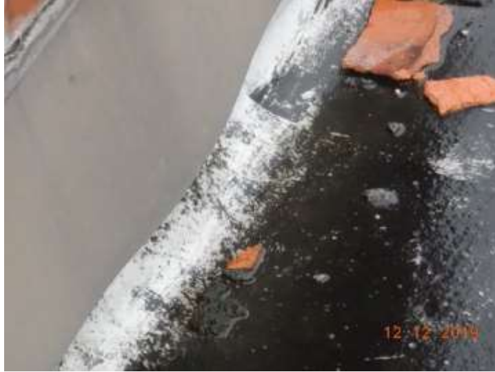
Masonry debris on the roof
