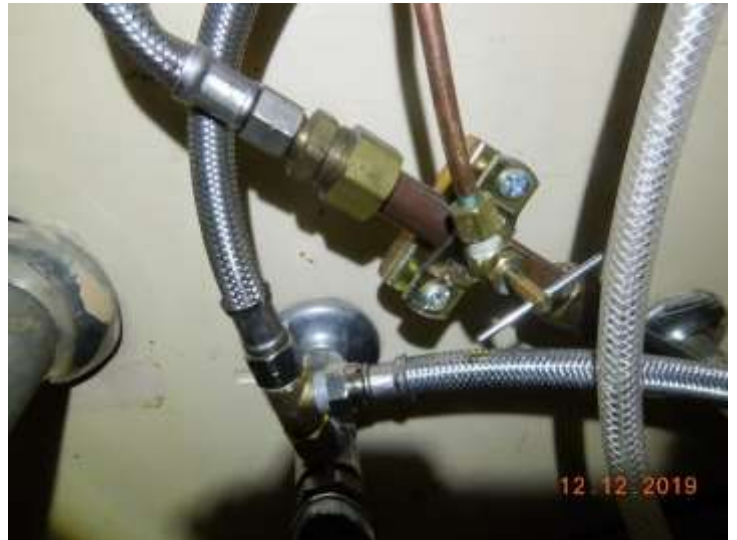
A shut off valve for the refrigerator water supply appears to be located in the sink base cabinet
