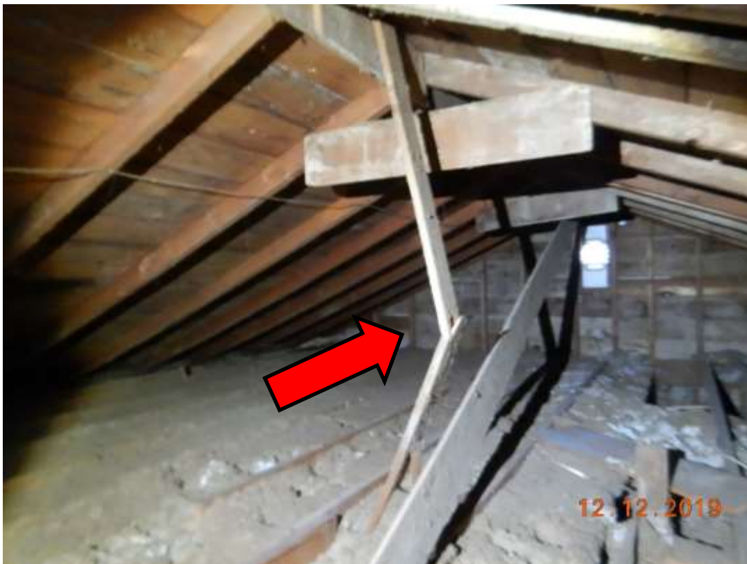
Cracked ridge post
