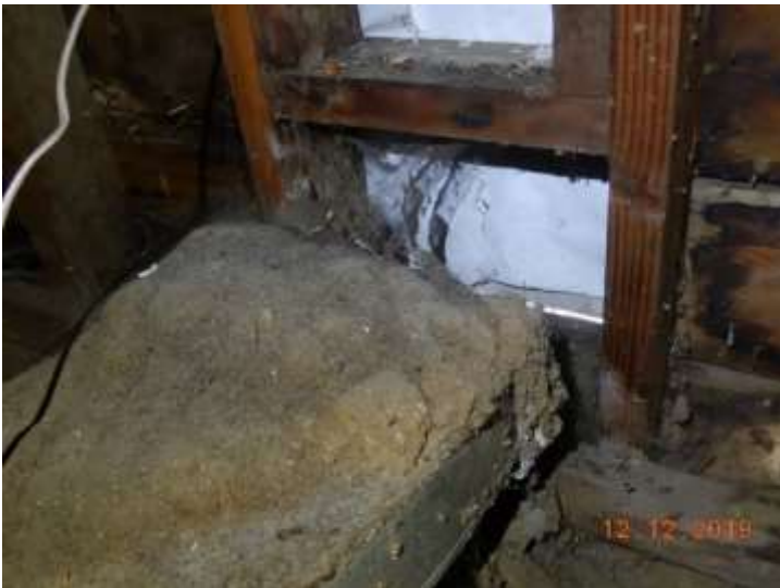
The kitchen vent does not extend to the exterior
