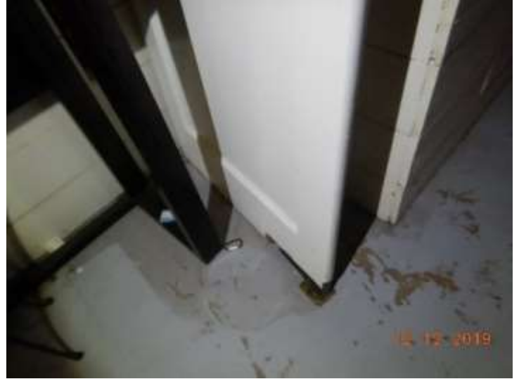
A stored door located in the basement appears to be the removed door from the Kitchen
