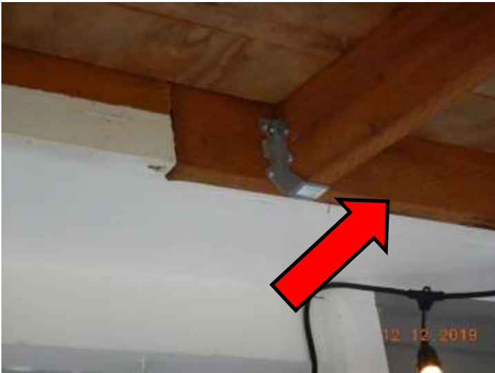
The ledger of the rear roof does not appear to be lag bolted to the home
