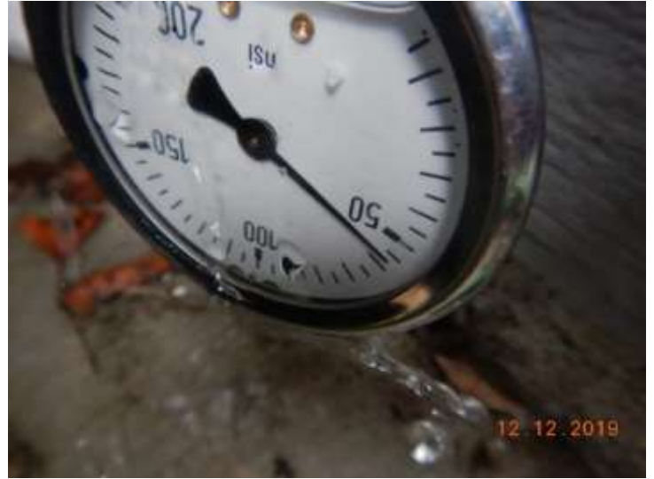
Water pressure is adequate and not excessive
